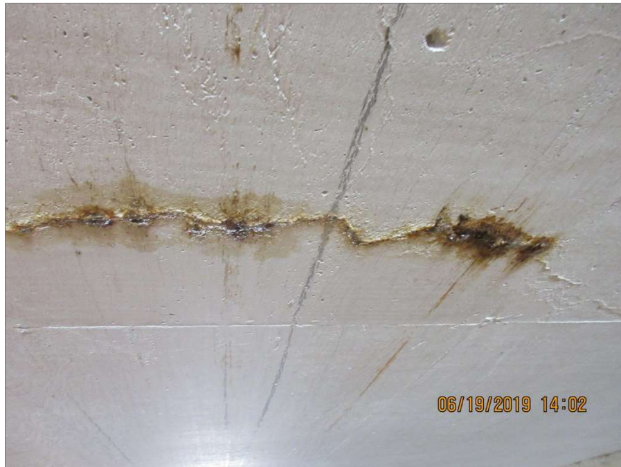
Photo 19.3 – Ceiling crack with rust stains and water intrusion at Tunnel #1.
