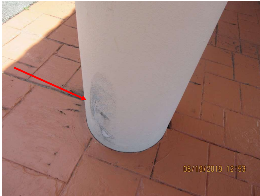
Photo 17.1 – Delaminated paint and impact marks on overhang structure column at Guard House #1
