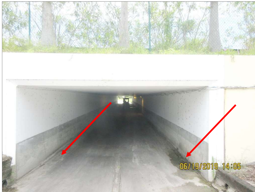
Photo 19.6 – Evidence of ponding/poor drainage at edges of Tunnel #1
