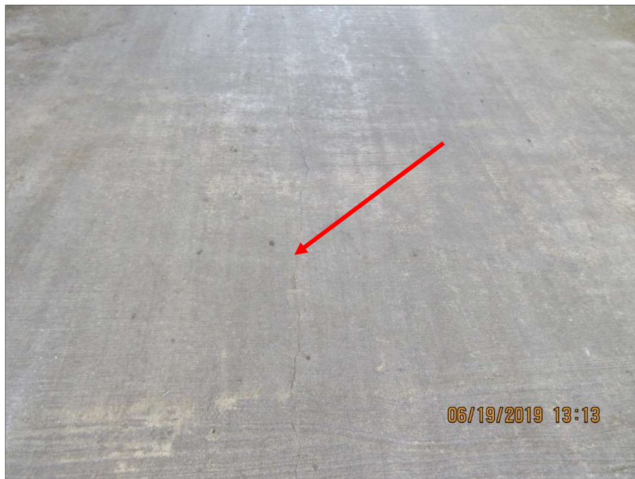
Photo 19.12 – Cracks in slab on grade of Tunnel #3
