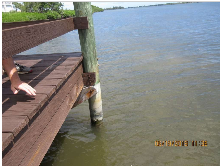
Photo 20.2 – Corrosion stains (rust) were visible at the anchor bolts for the cross bracing of River Village Pier
