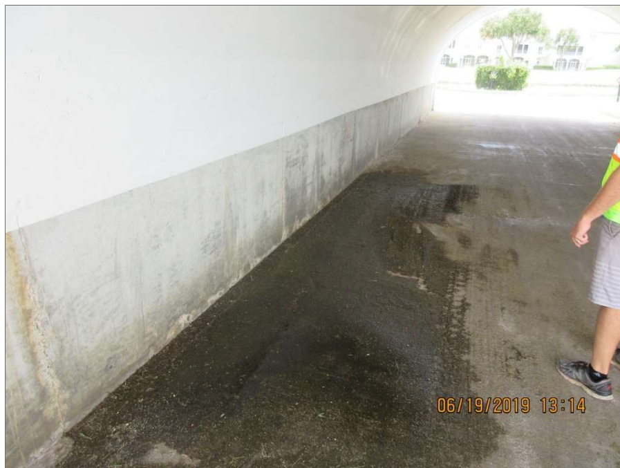
Photo 19.14 – Evidence of ponding/poor drainage at Tunnel #3
