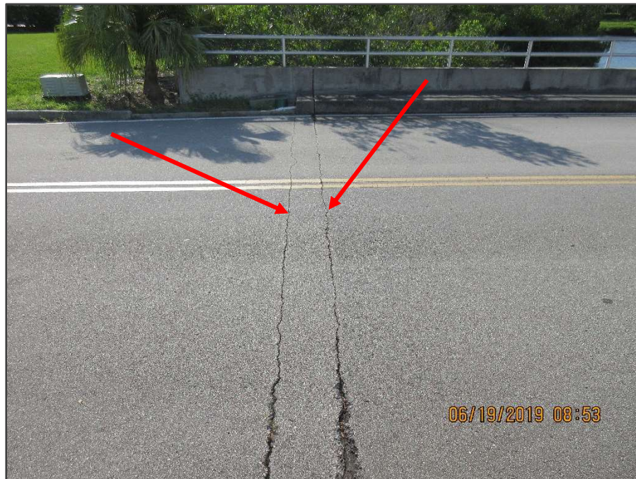
Photo 16.1 – Cracking at bridge #2 approach
