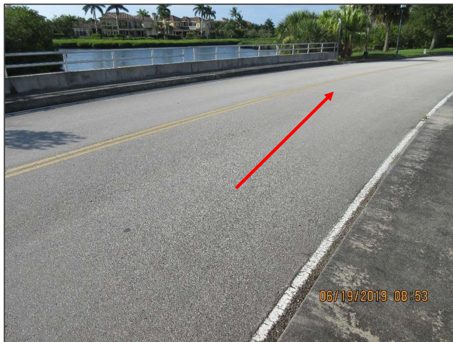
Photo 16.2 – Transverse crack at mid-span of bridge #2
