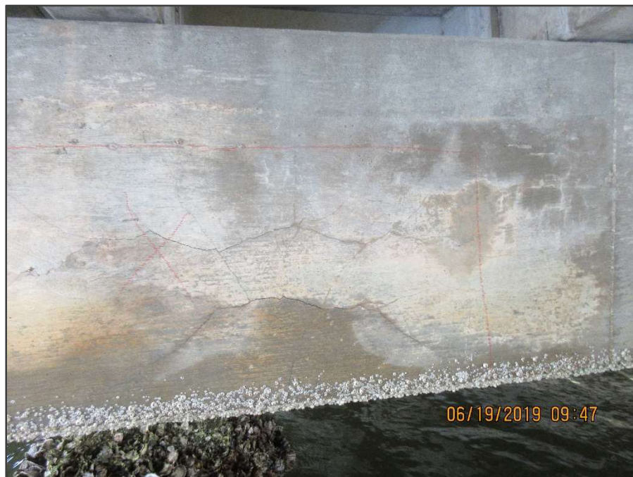
Photo 16.8 – Cracking on intermediate bent of bridge #2. Note vegetative growth on bent and piles (typical throughout)
