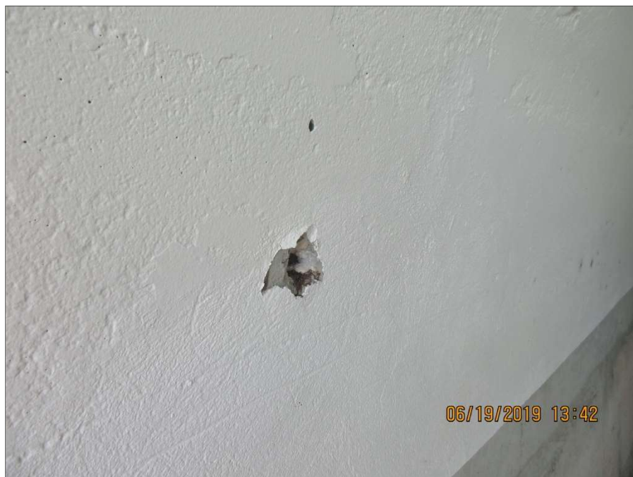
Photo 19.10 – Localized concrete spall in wall of Tunnel #2
