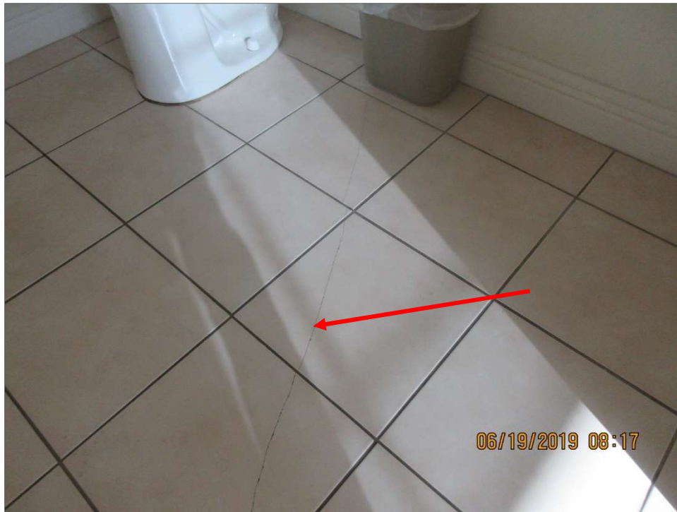
Photo 17.7 – Cracking on bathroom floor tiles at Guard House #2
