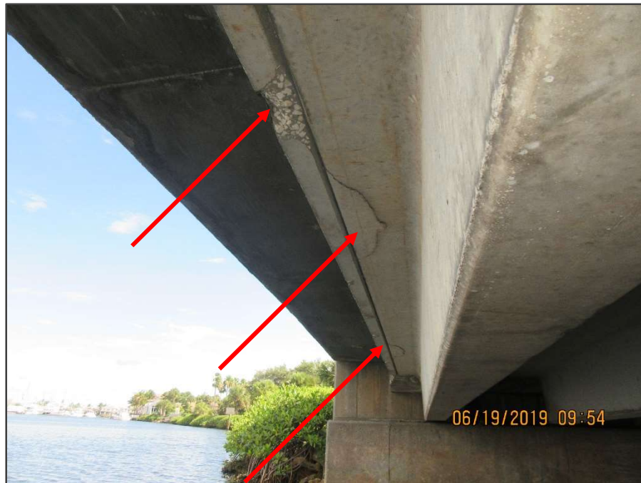
Photo 16.9 – Concrete spalls on the flange and fascia of the exterior Double-T beams at bridge #2
