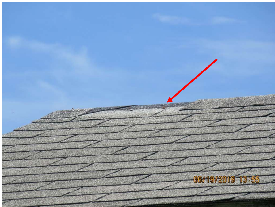
Photo 20.8 – Missing shingle at Guard Shack
