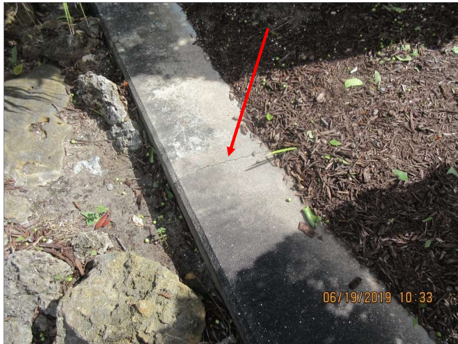
Photo 18.10 – Transverse crack on the cap of Retaining wall Span #2
