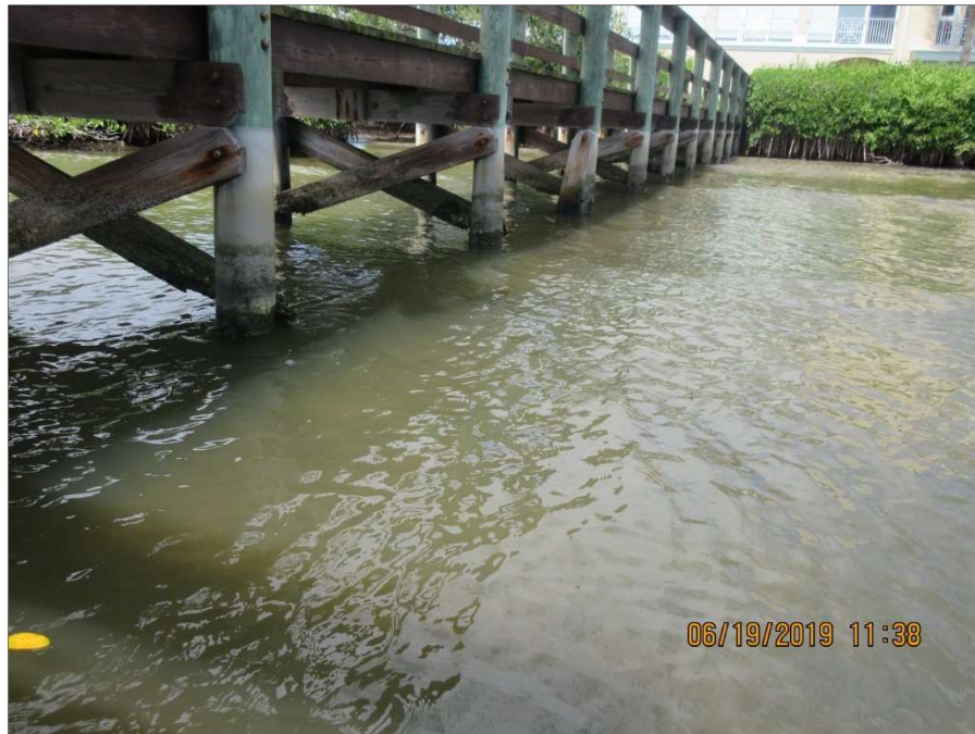
Photo 20.3 – The 2x8 timber cross bracing was rotted, splintered & deteriorated throughout.
