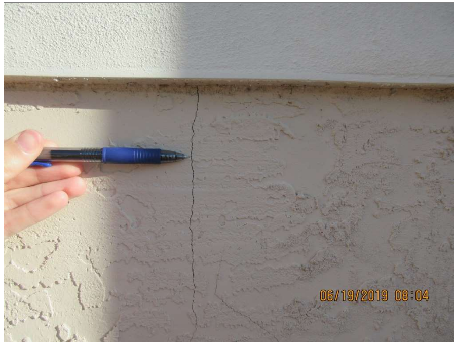
Photo 17.5 – Stucco crack on Guard House #2 (typical throughout)
