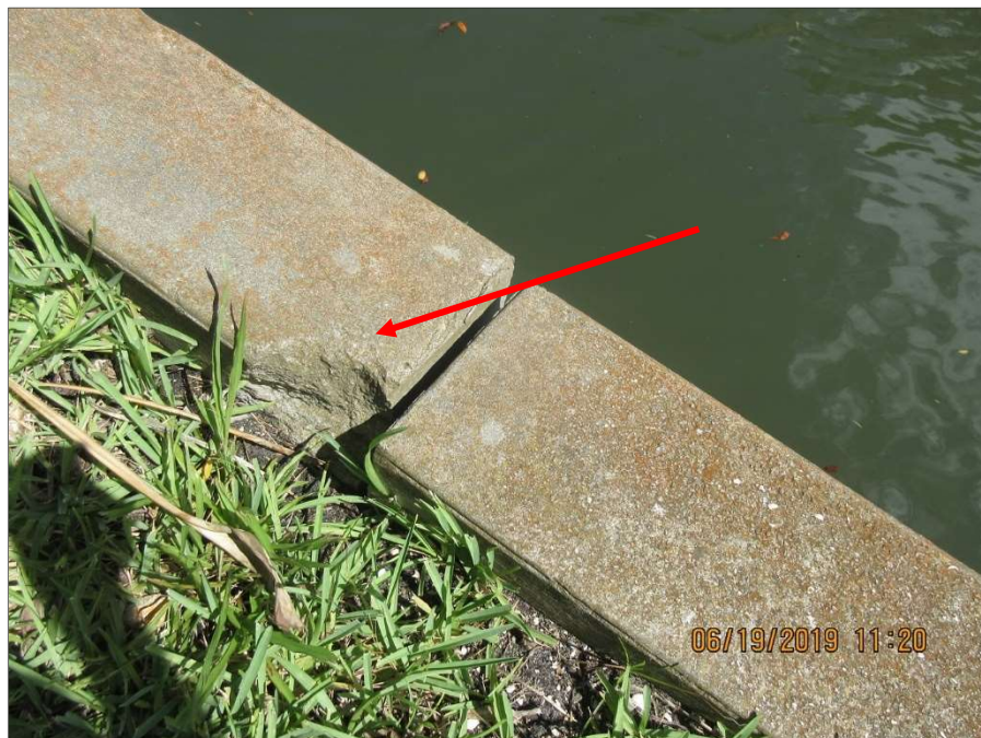
Photo 18.5 –Localized concrete damage to edge of retaining wall cap at Retaining wall Span #1
