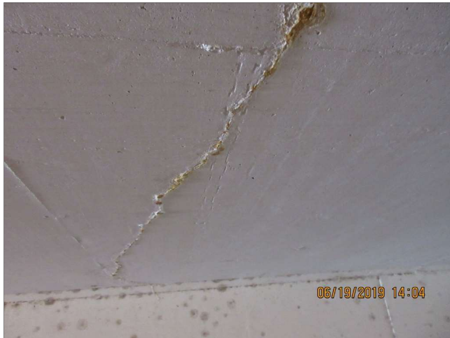
Photo 19.4 – Ceiling crack with rust stains and water intrusion at Tunnel #1.
