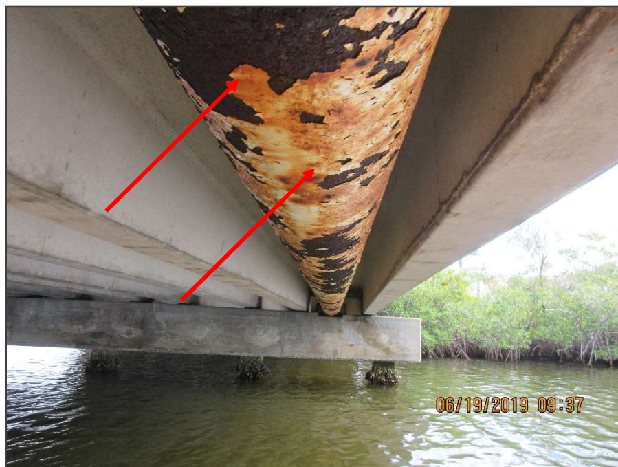
Photo 16.6 – Corrosion observed on the utility pipe spanning the length of the bridge under bridge #2
