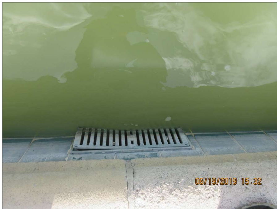
Photo 20.12 – Bent skimmer in fountain
