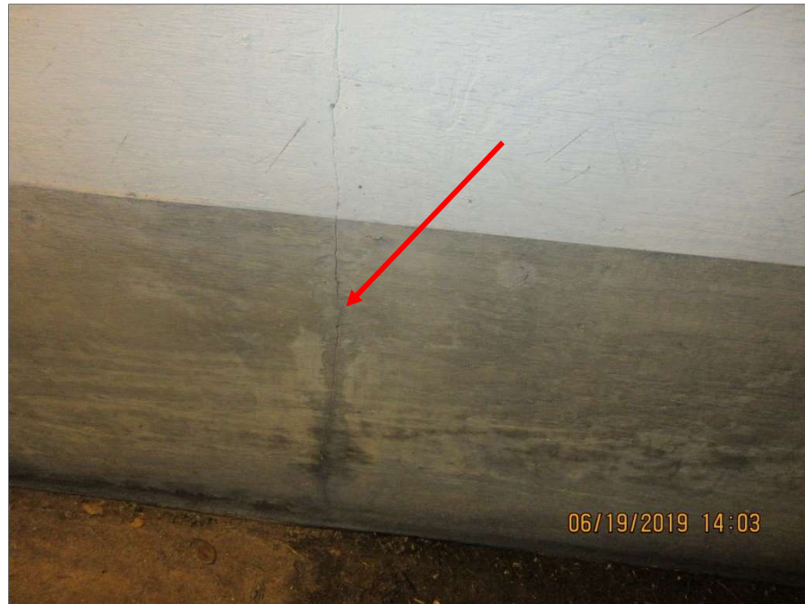
Photo 19.7 – Crack in wall of Tunnel #1
