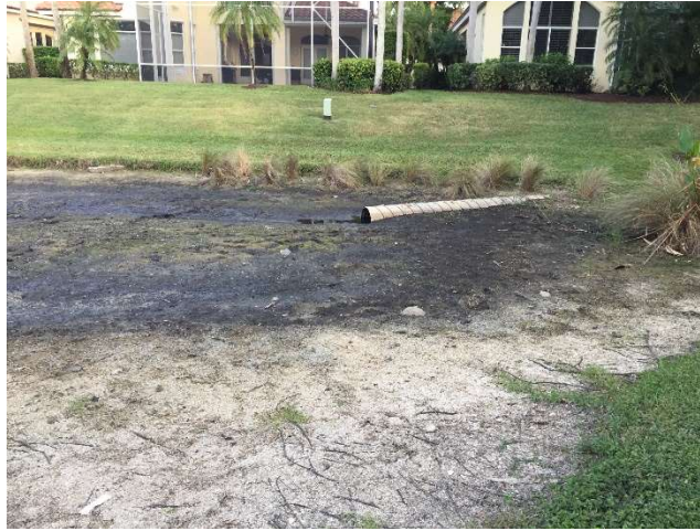
Photo 8.3 – Siltation in Pond #16
