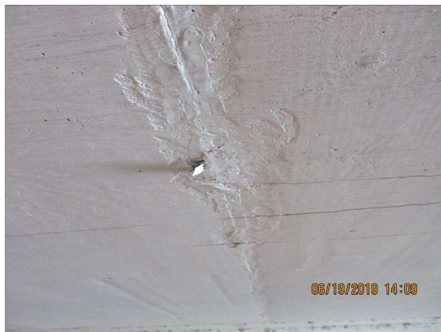
Photo 19.2 –Paint delamination of the ceiling of Tunnel #1
