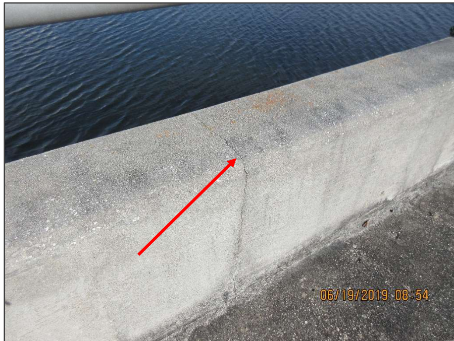
Photo 16.5 – Cracks in the concrete barrier wall (typical throughout) at bridge #2
