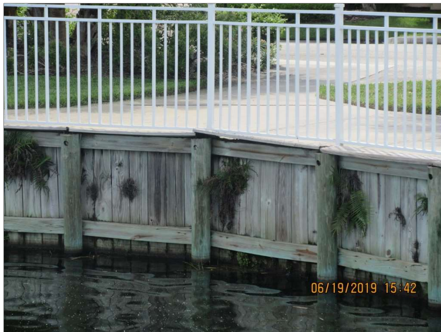
Photo 18.12 – Vegetation growing on retaining wall #3
