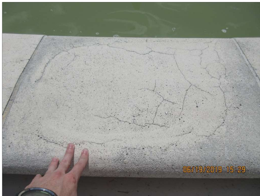
Photo 20.10 – Cracking on coping of Fountain
