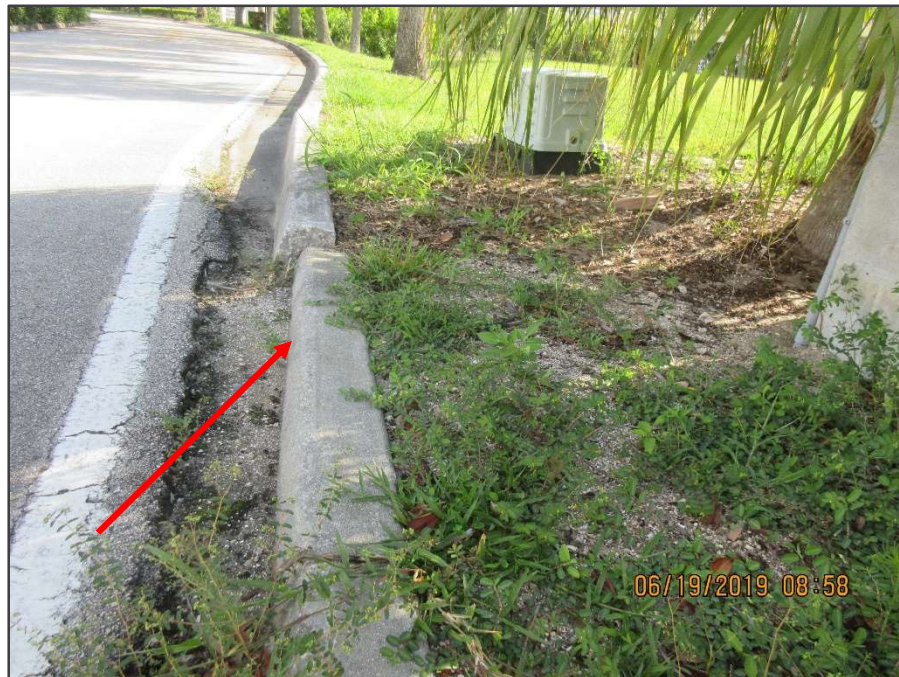
Photo 16.3 – Deflection of the curb and gutter at approach to bridge #2
