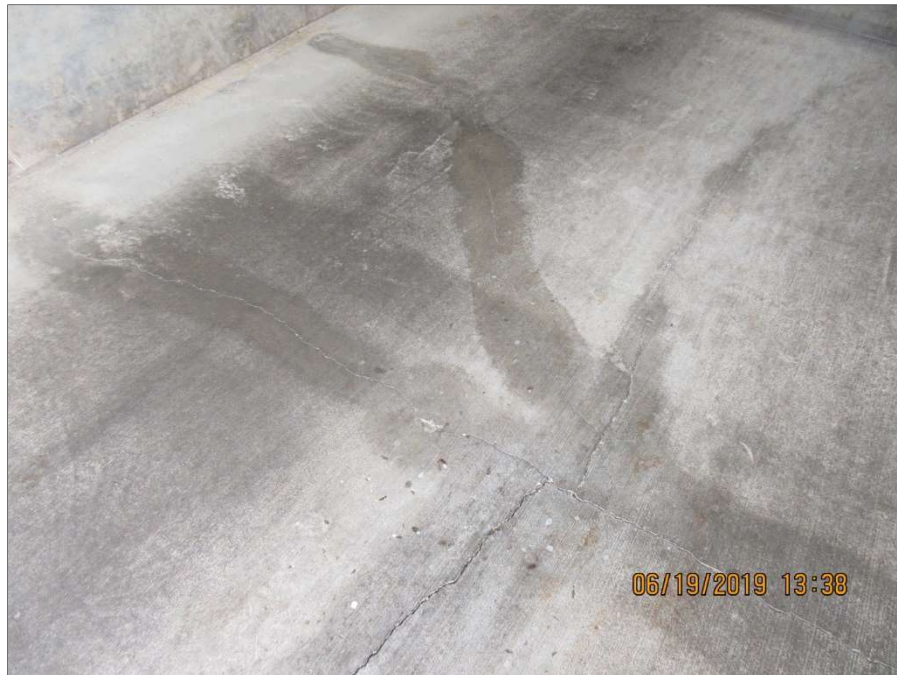
Photo 19.9 – Cracks in topping slab at Tunnel #2 (typical throughout)
