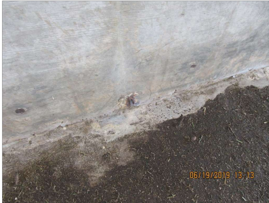
Photo 19.13 – Exposed reinforcing in wall on Tunnel #3
