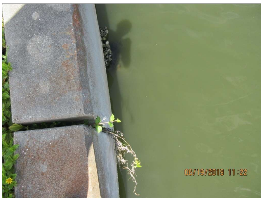
Photo 18.7 –Vegetation observed at joints in Retaining wall Span #1
