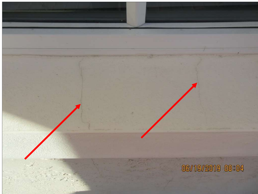
Photo 17.6 – Stucco crack on window sill ledge at Guard House #2 (typical throughout)
