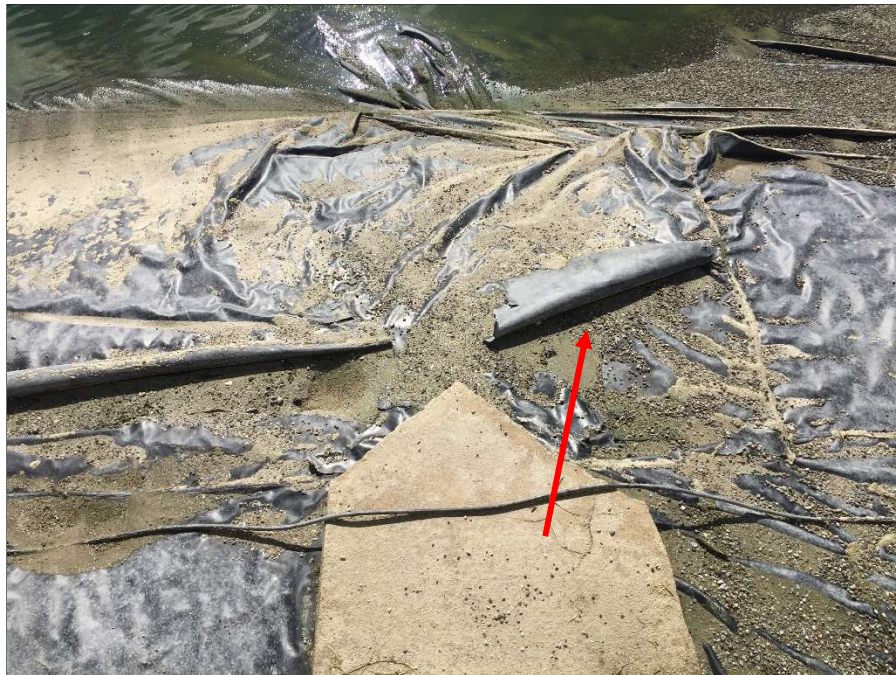
Photo 18.25 – Pond liner in the recycled water reservoir with tears
