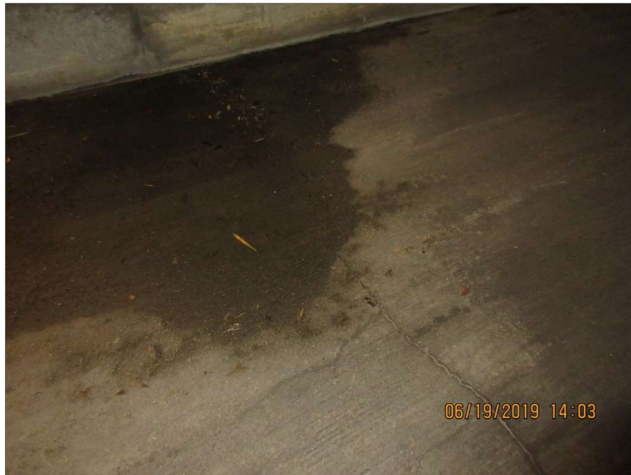
Photo 19.5 – Evidence of ponding/poor drainage and crack in slab in Tunnel #1
