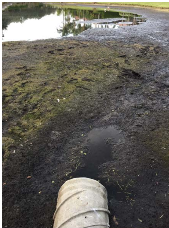
Photo 8.4 – Siltation in Pond #16
