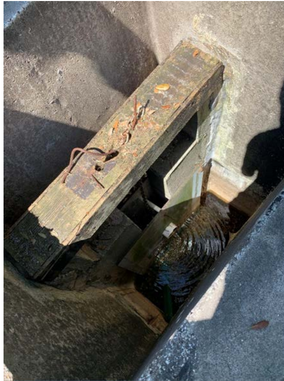
Photo 8.5 – Un-permitted control structure
