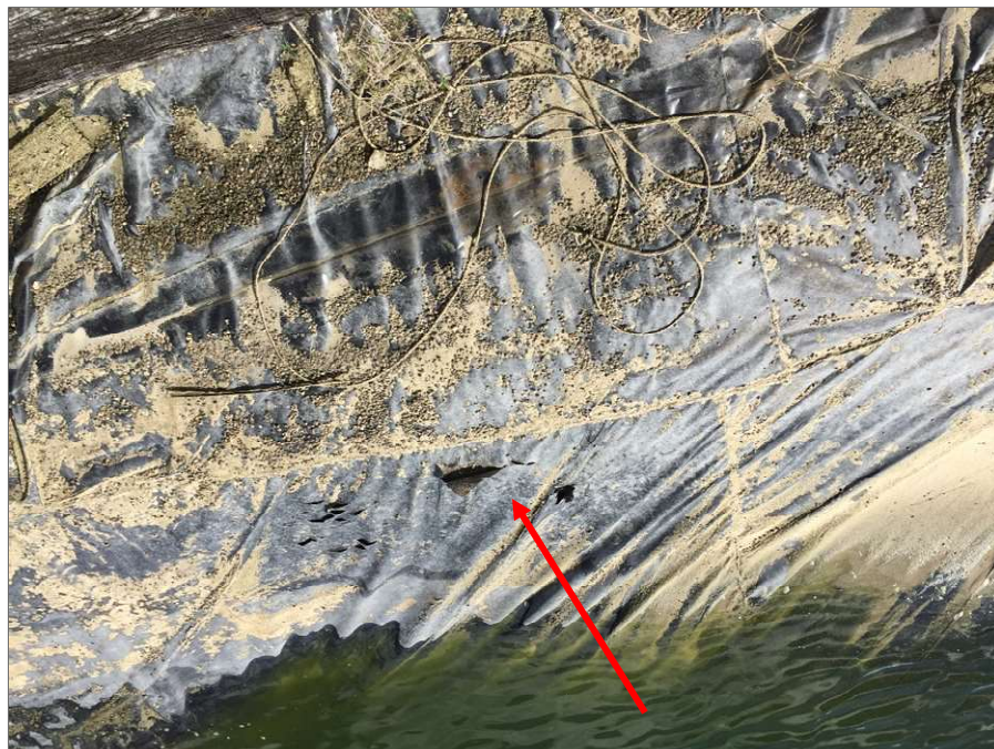
Photo 18.23 – Pond liner in the recycled water reservoir with tears.
