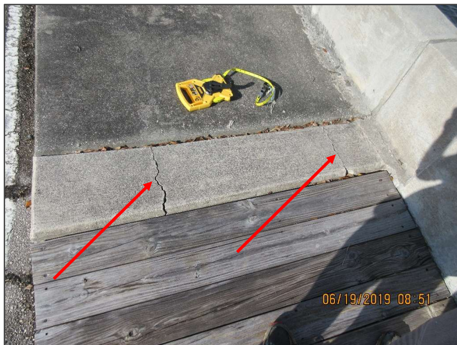
Photo 16.4 –Cracking in the abutment wall at the elevation of the sidewalk at bridge #2
