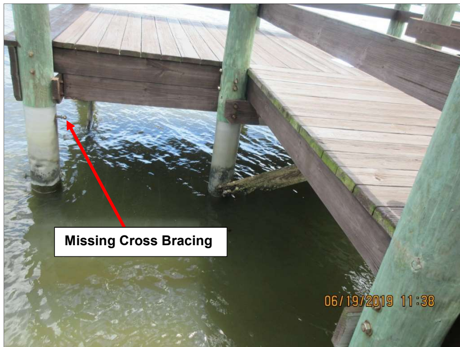
Photo 20.4 – The 2x8 timber cross bracing was rotted, splintered, deteriorated and/or missing throughout.
