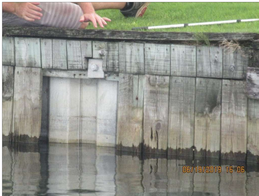
Photo 18.15 –Missing timber boards on Retaining wall Span #4
