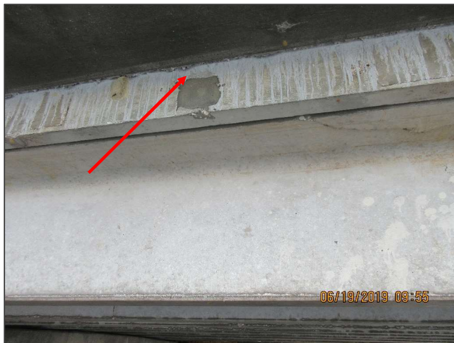
Photo 16.10 – Concrete spalls on the Double-T beam fascia at the post tension grout pockets at bridge #2
