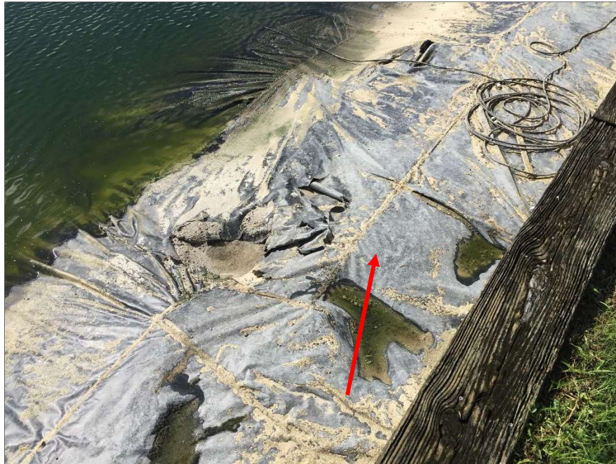
Photo 18.24 – Pond liner in the recycled water reservoir with tears.
