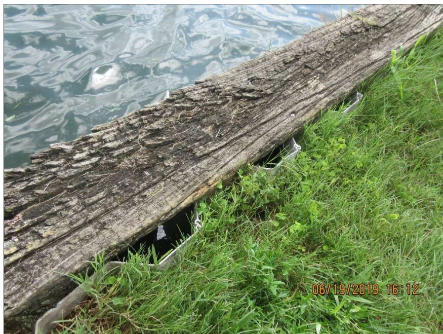
Photo 18.19 –Cracking splintering and displacement of timber boards on Retaining wall Span #4
