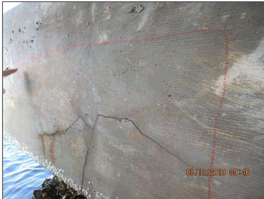
Photo 16.7 – Cracking on the intermediate bent on both north and south sides of bridge #2
