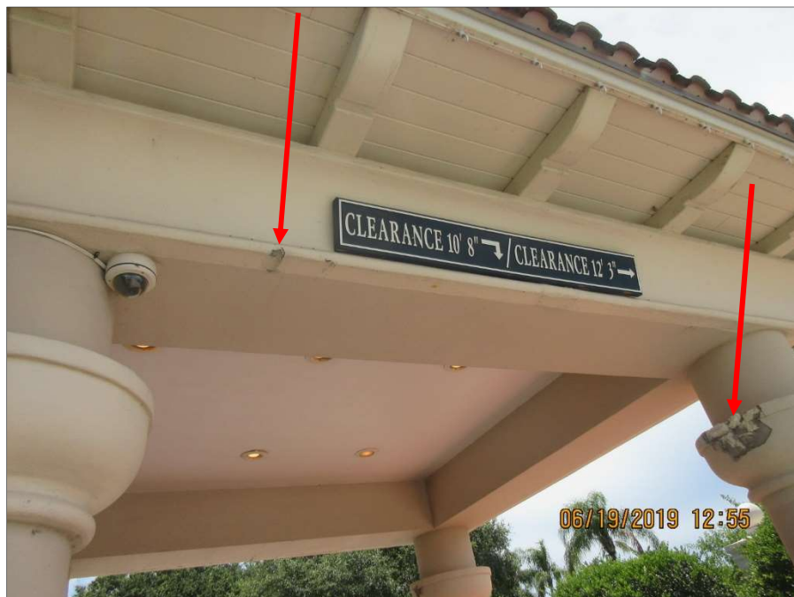
Photo 17.2 – Exposed stucco lath on overhead beam; damage to architectural feature on column at Guard House #1
