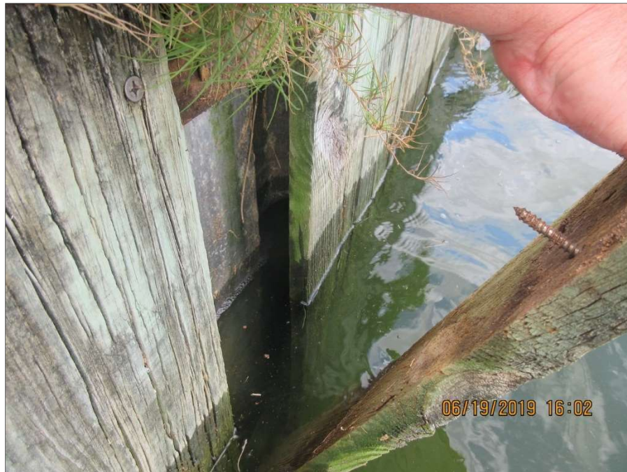
Photo 18.16 –Missing timber boards on Retaining wall Span #4
