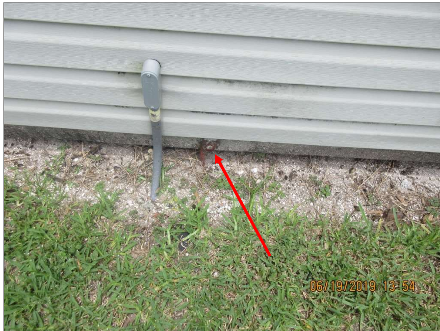
Photo 20.6 – Corroded anchor at Via Marbella Guard Shack
