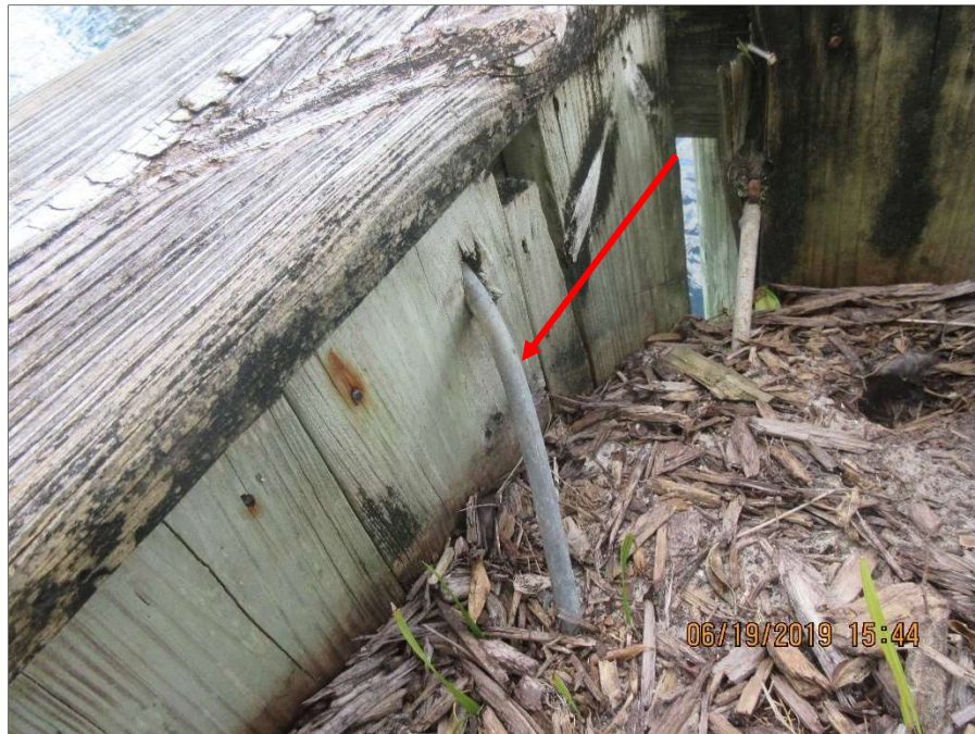
Photo 18.14 – Bent tie back rod at Wall #3
