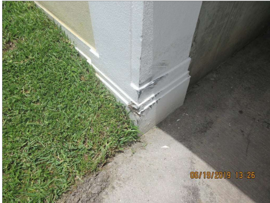
Photo 19.15 – Evidence of impact damage to the base of the arch at the entry to Tunnel #4
