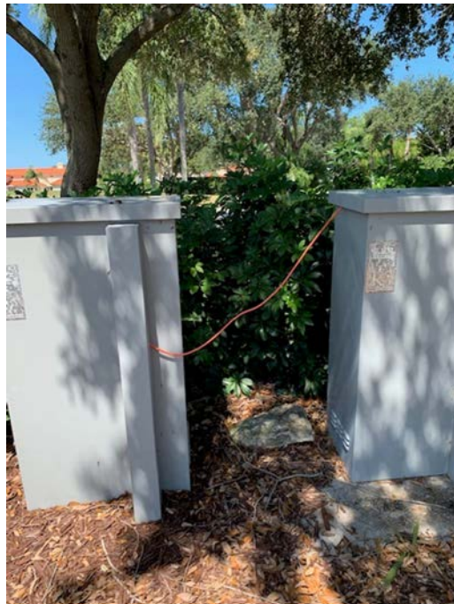
Photo 6.3 - Exposed wire coming from the electrical box near Saint David's.
