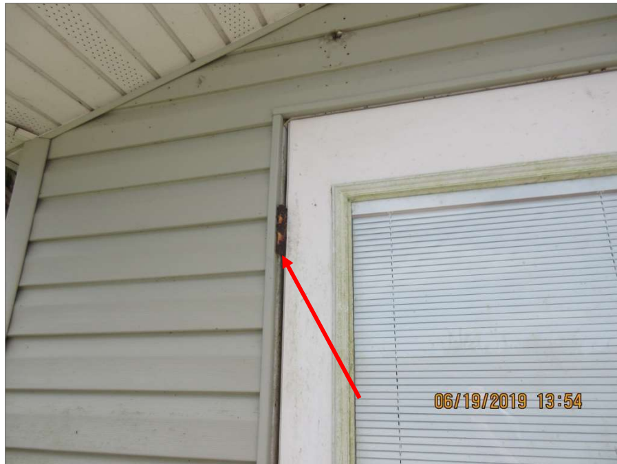
Photo 20.7 – Corroded door hinges at Guard Shack
