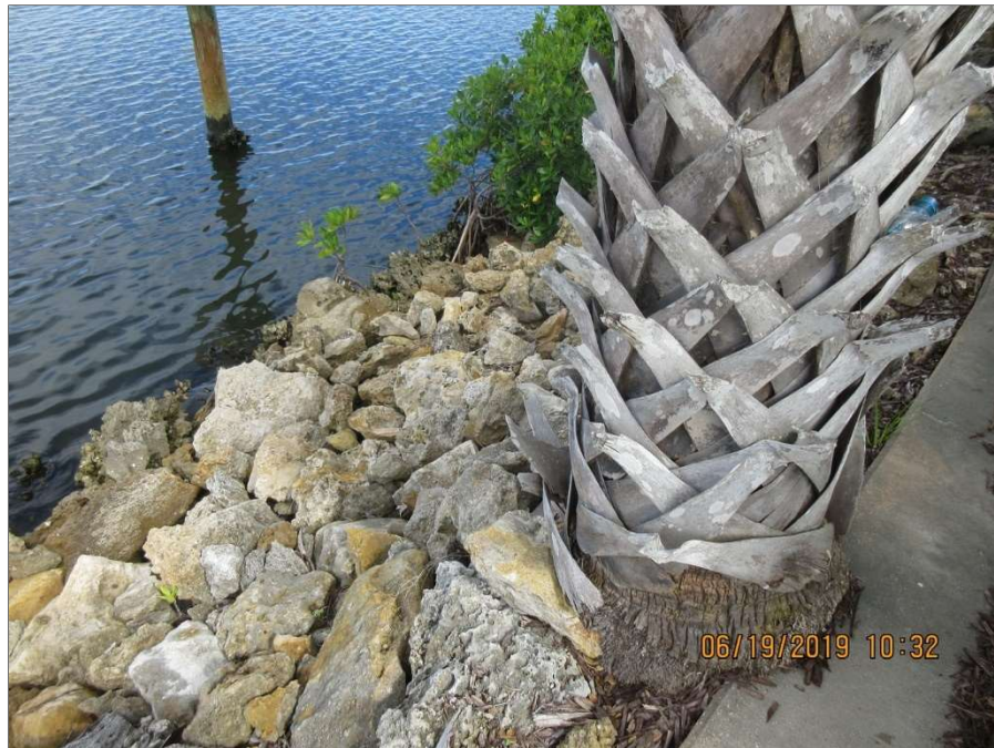
Photo 18.8 –Palm encroaching on Retaining wall Span #2
