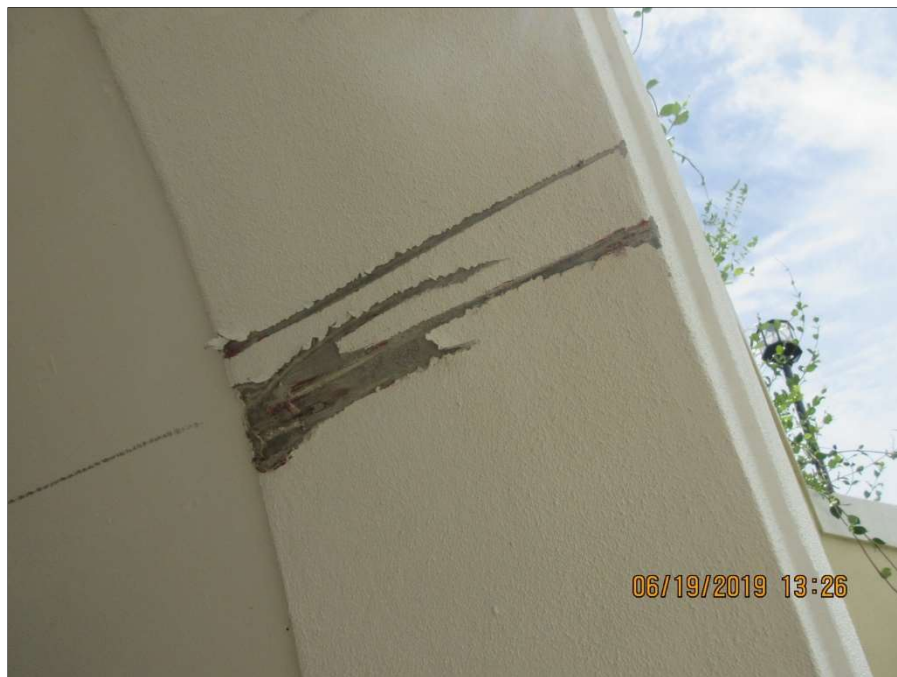
Photo 19.15 – Evidence of impact damage to the arch at the entry to the Tunnel #4
