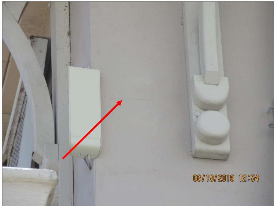
Photo 17.3 – Stucco crack on Guard House #1
