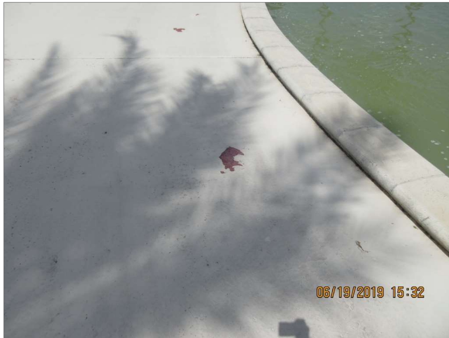
Photo 20.11 – Delamination of finish on sidewalk surrounding fountain
