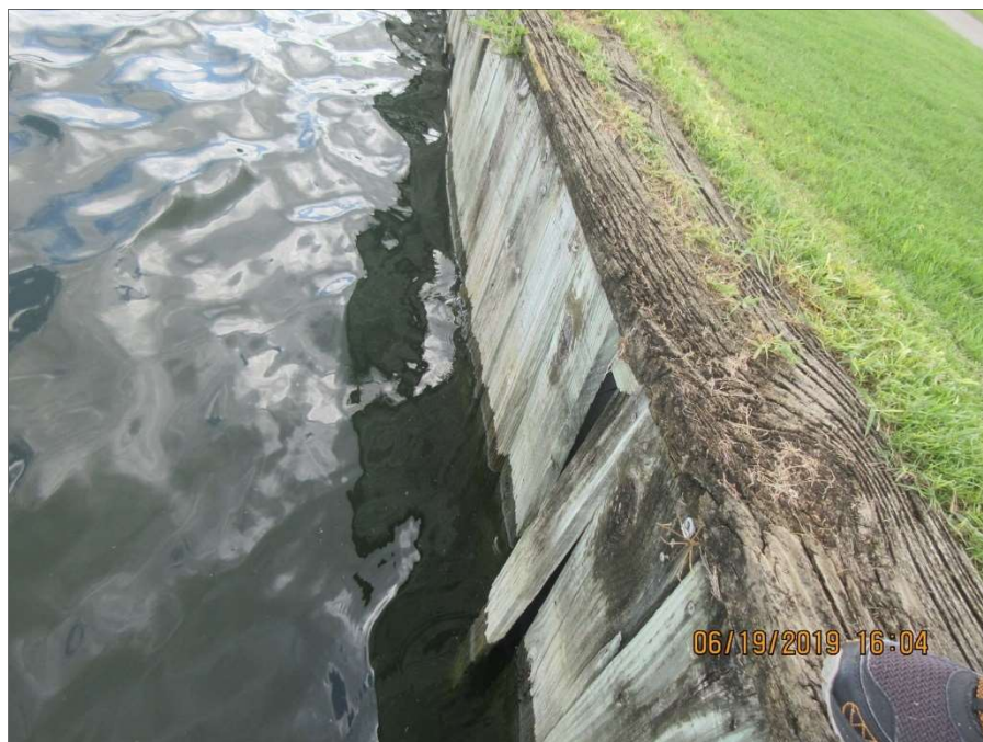
Photo 18.17 –Damaged and rotting timber boards on Retaining wall Span #4
