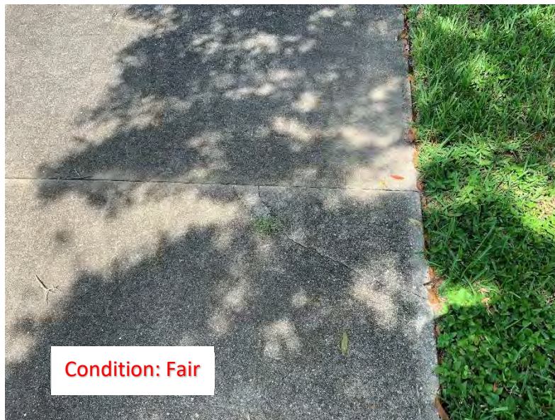
(254) Center and Corner Cracks (7)
