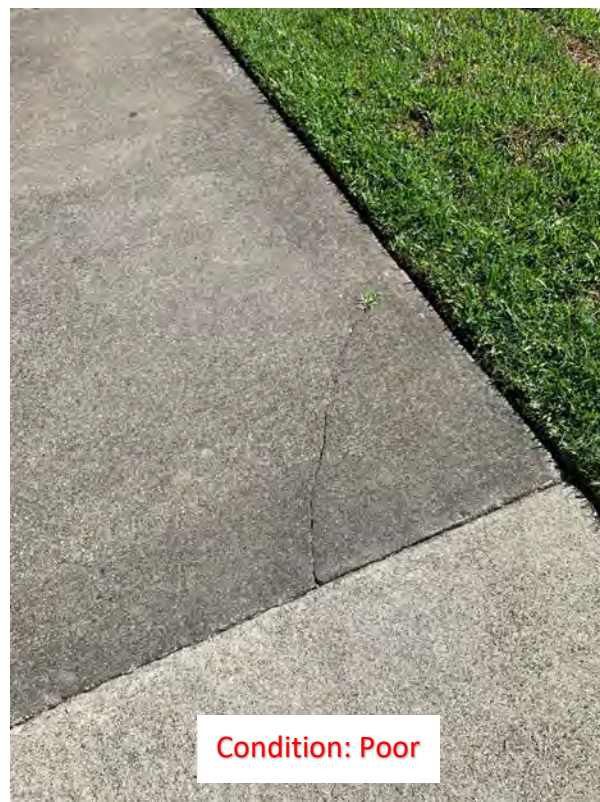
(242) Elevated Corners and Corner Crack (2)
