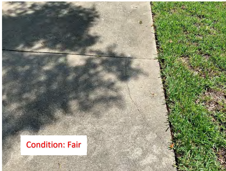
(254) Center and Corner Cracks (2)
