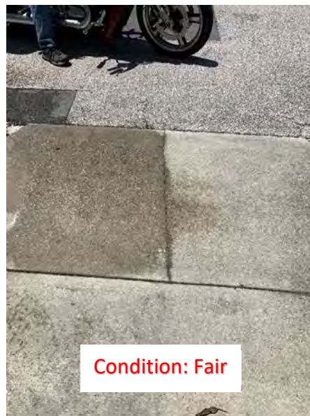
(295) Center and Corner Cracks (2)
