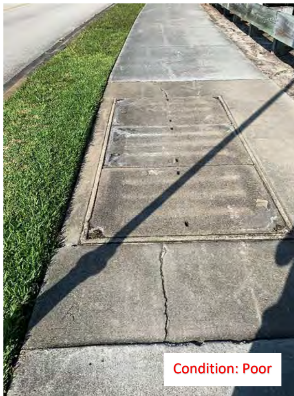
(188) Elevated Corners and Center Cracks
