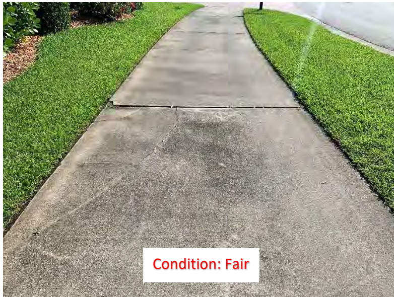
(226) Elevated Corner and Large Corner Cracks
