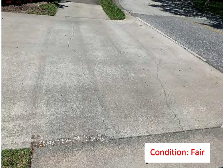
(285) Center Cracks and Chipped Concrete
