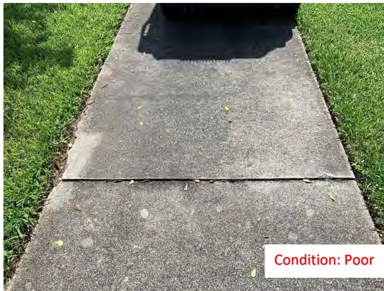
(260) Elevated Corner and Chipped Concrete
