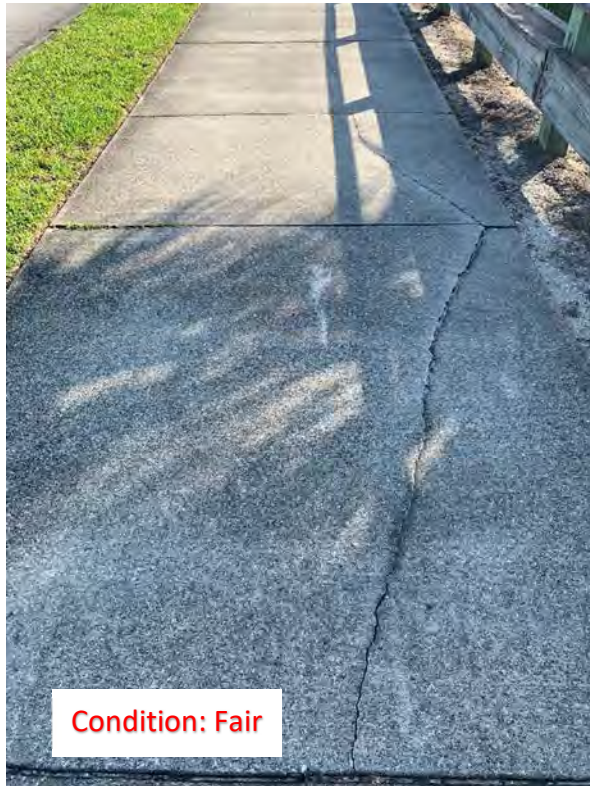
(166) Large Corner Cracks
