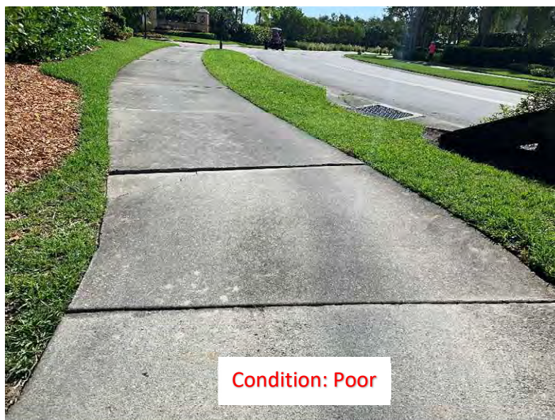
(224) Elevated Corners and Corner Cracks
