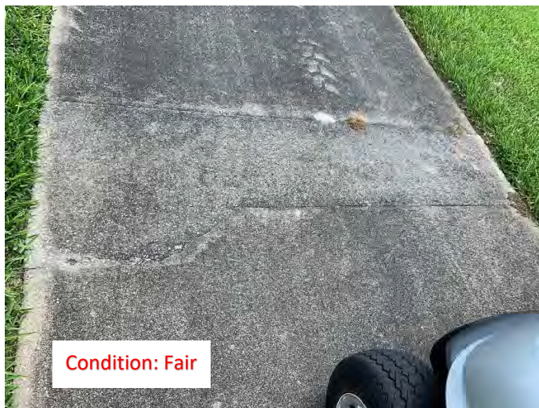
(254) Center and Corner Cracks (1)
