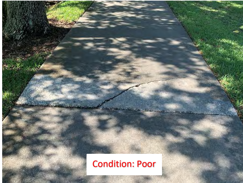
(240) Elevated Corners and Corner Cracks
