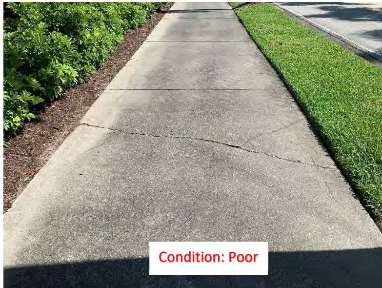
(243) Elevated Corners, Corner Cracks and Large Center Cracks (1)
