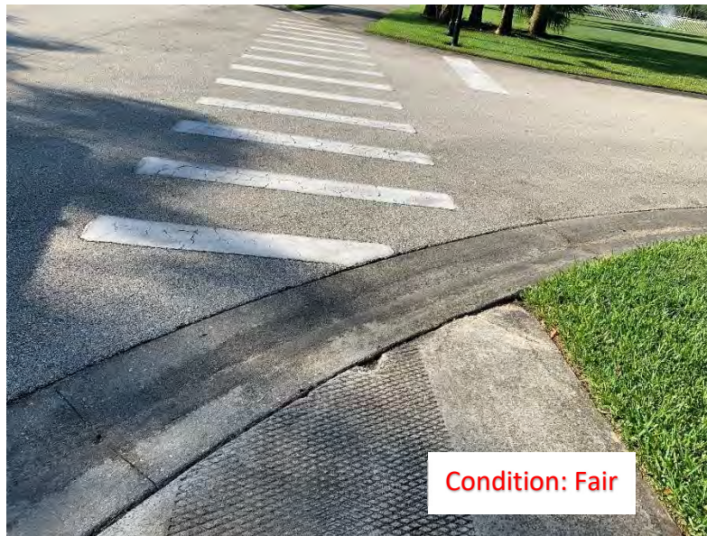
(183) Corner Crack and Chipped Concrete
