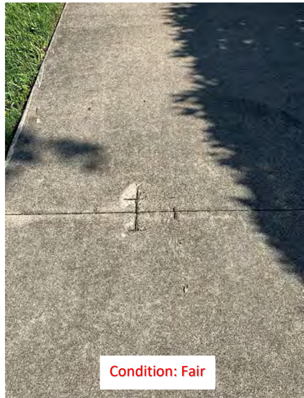
(213) Chipped Concrete Areas (2)
