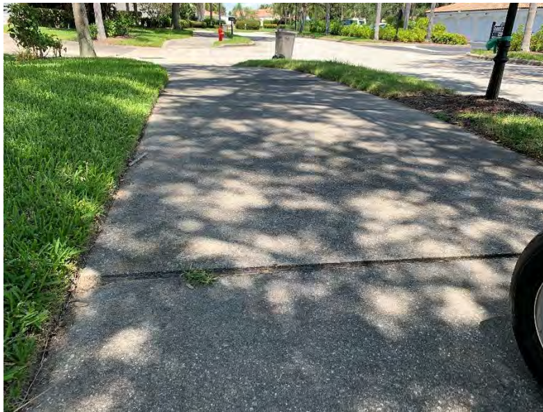
(284) Elevated Corners and Center Cracks (3)
