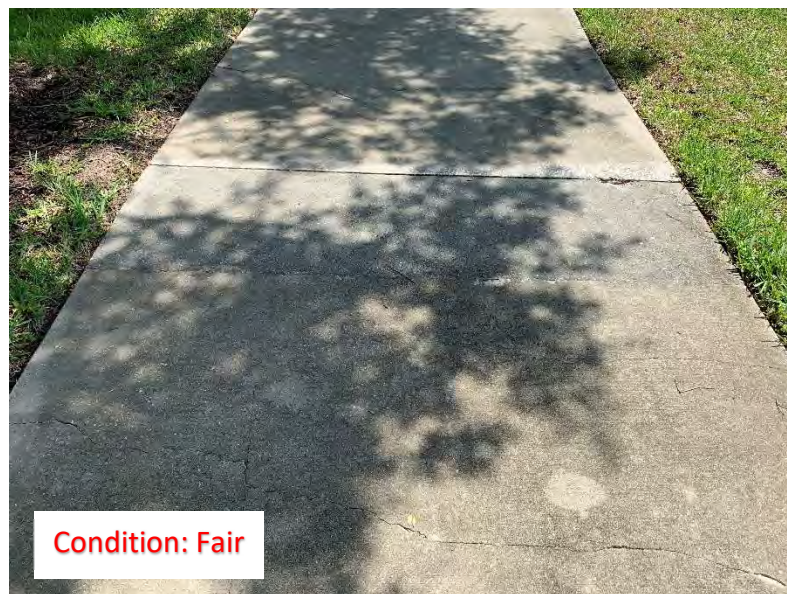
(254) Center and Corner Cracks (5)
