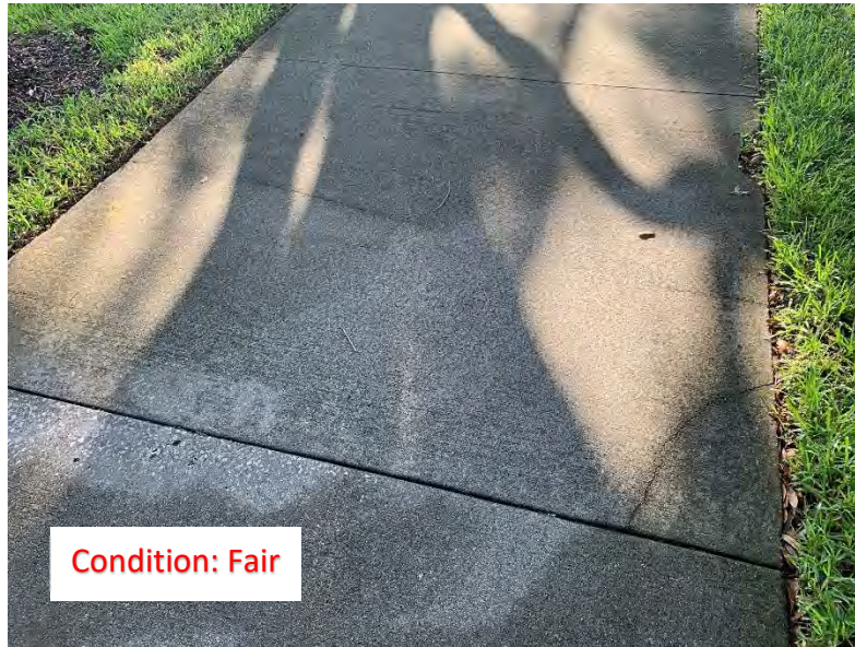
(155) Center and Corner Cracks
