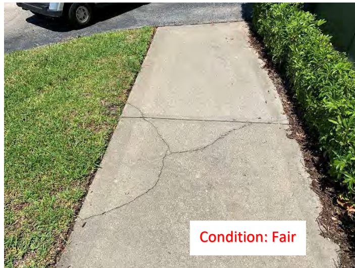
(295) Center and Corner Cracks (1)
