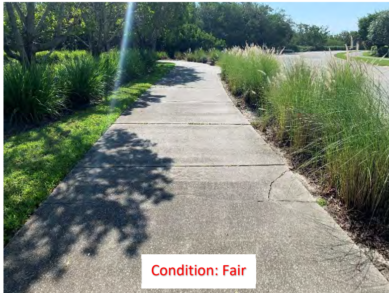
(229) Center and Corner Cracks
