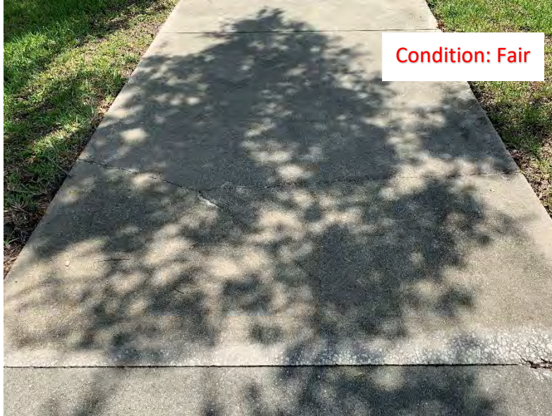
(254) Center and Corner Cracks (6)
