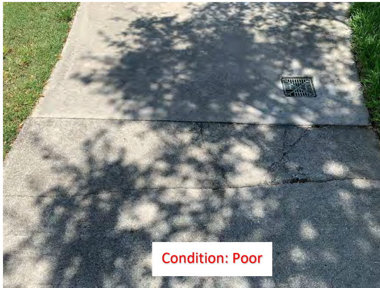
(303) Center and Corner Cracks
