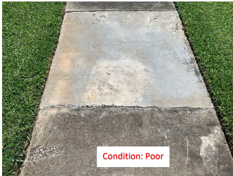
(262) Chipped Concrete, Corner Cracks and Center Cracks
