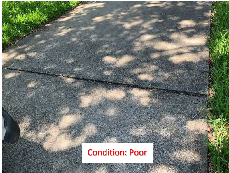
(291) Elevated Corners and Center Cracks (1)
