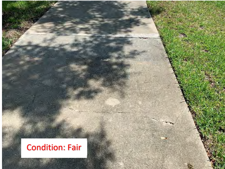
(254) Center and Corner Cracks (4)
