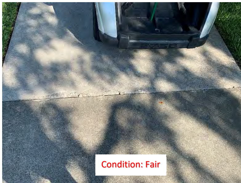
(207) Elevated Corners and Chipped Concrete
