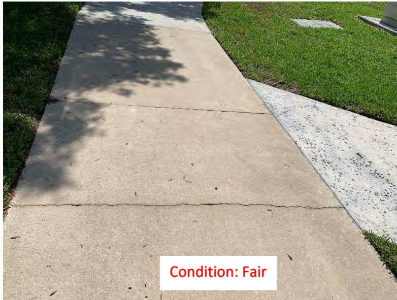
(250) Elevated Corners, Corner Cracks and Center Cracks (2)
