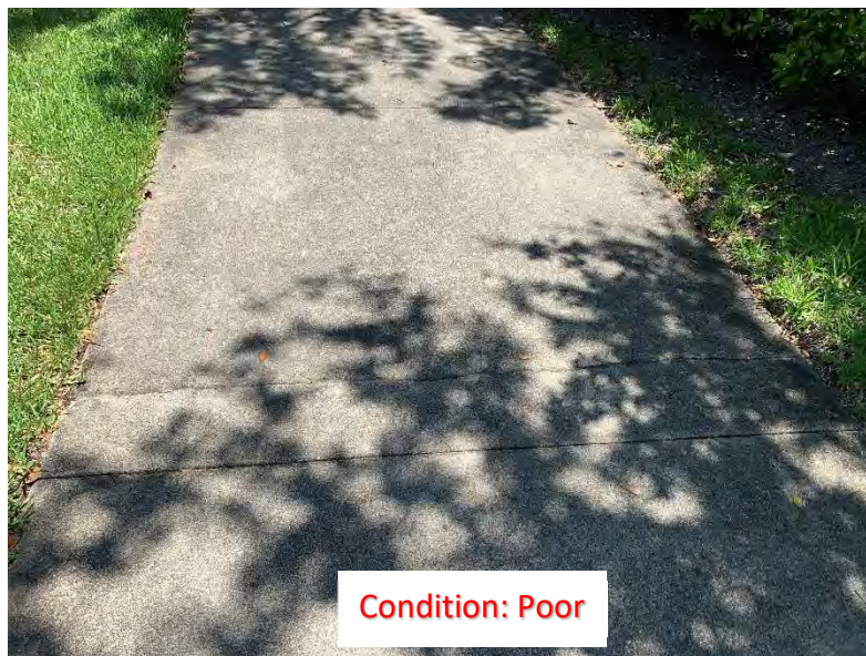
(291) Elevated Corners and Center Cracks (2)
