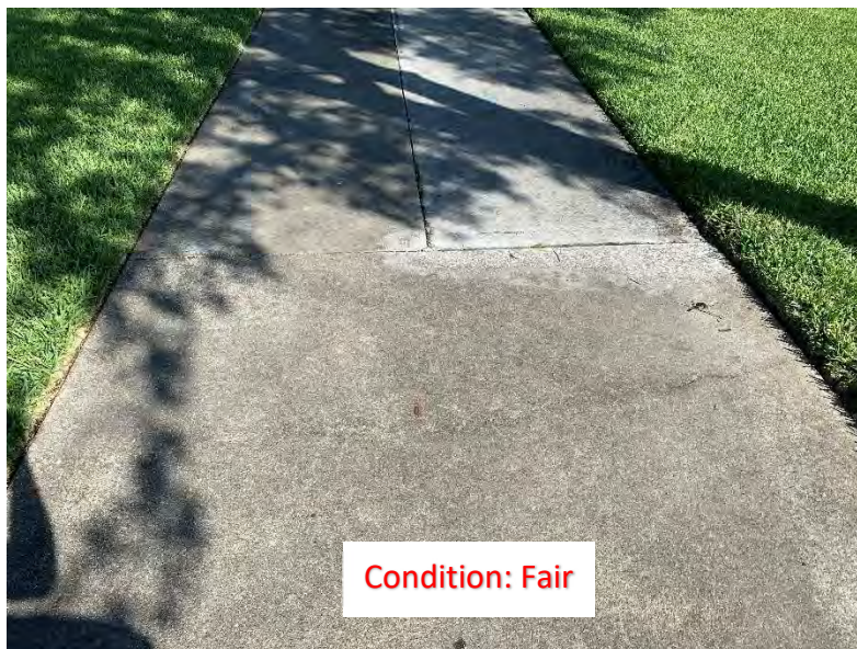
(205) Elevated Corner and Center Crack
