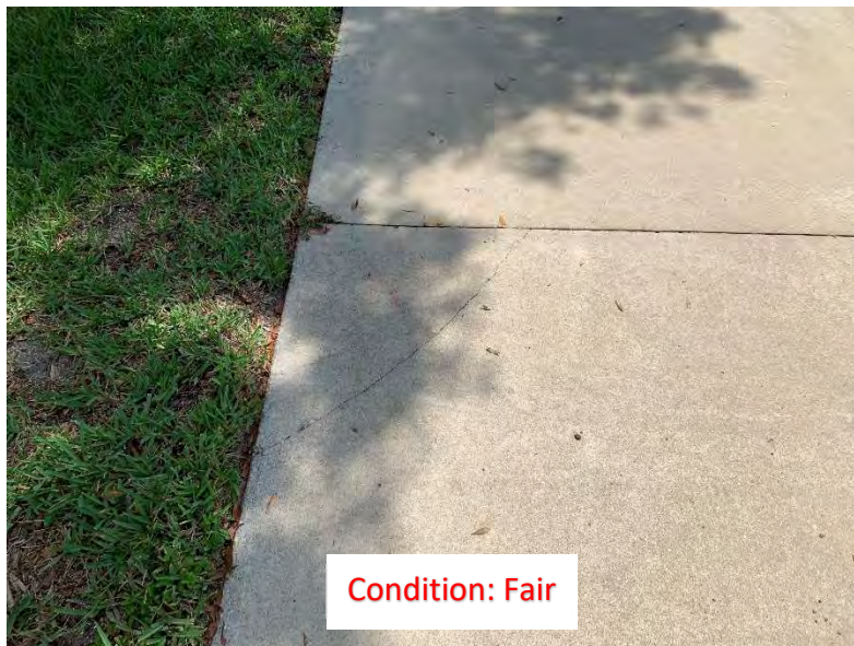
(250) Elevated Corners, Corner Cracks and Center Cracks (3)
