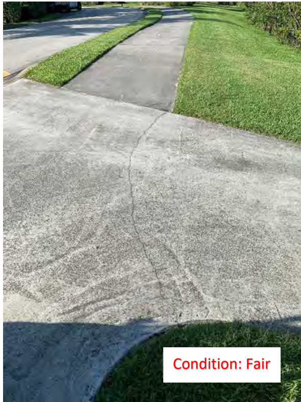
(178) Large Center Crack
