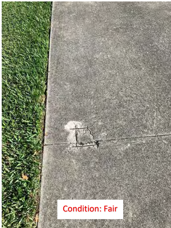
(213) Chipped Concrete Areas (1)
