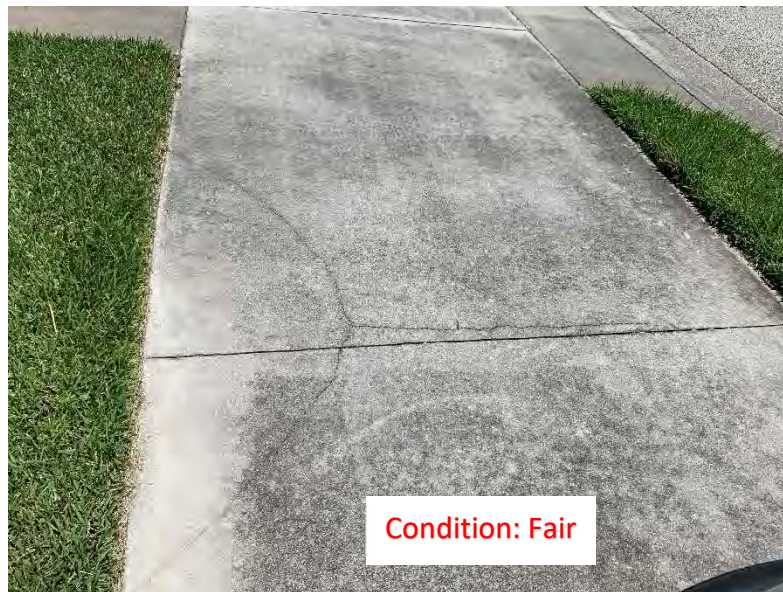
(286) Center and Corner Cracks
