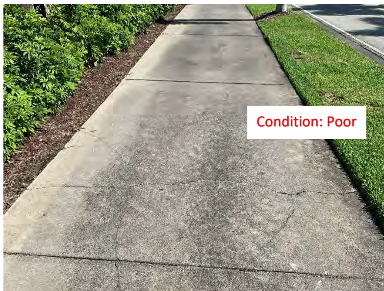
(243) Elevated Corners, Corner Cracks and Large Center Cracks (2)
