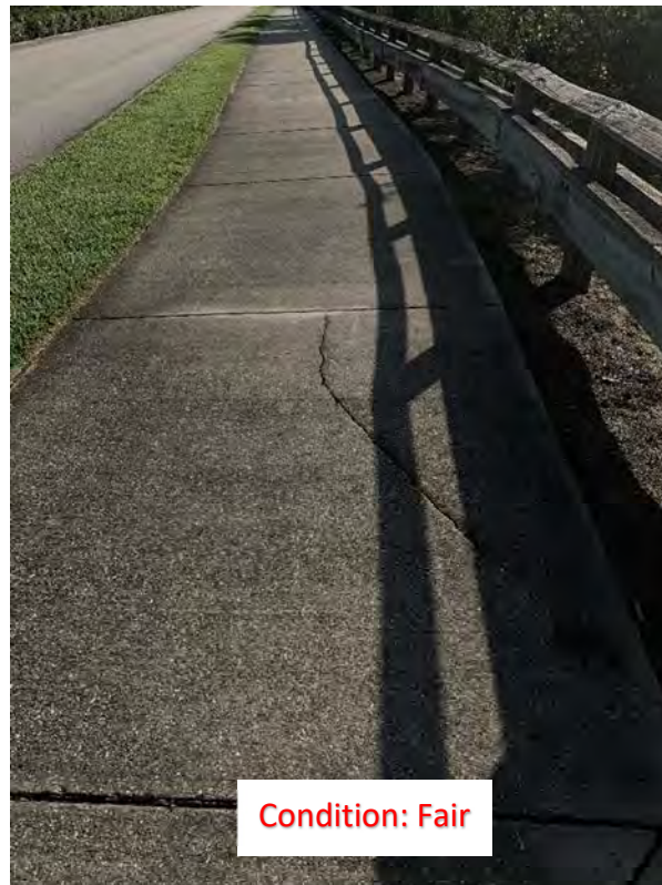
(163) Large Corner Cracks (2)
