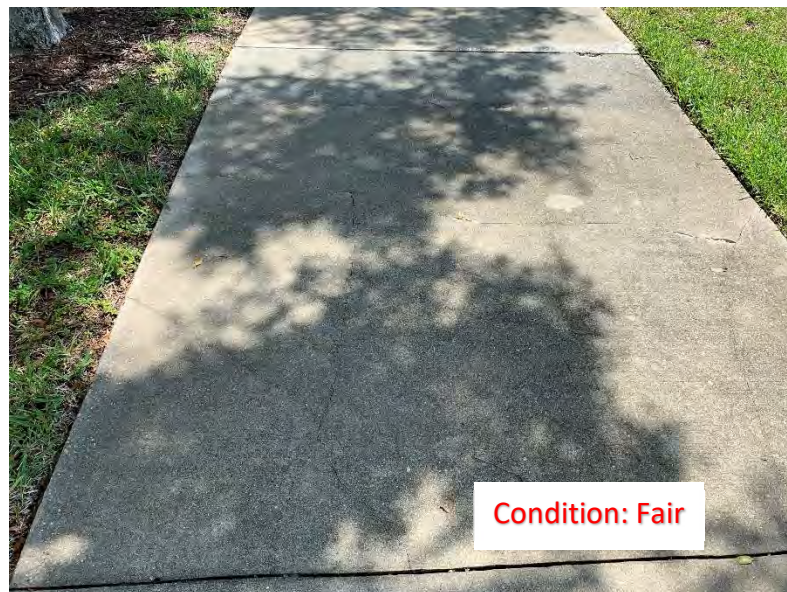
(254) Center and Corner Cracks (3)
