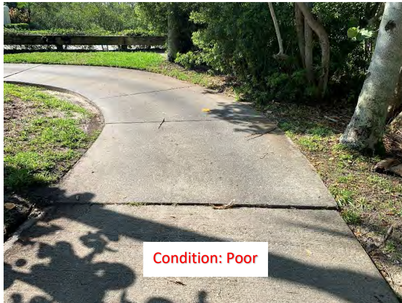
(223) Elevated Corners and Corner Cracks
