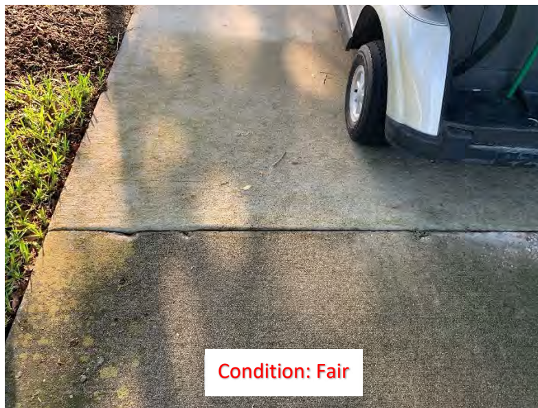
(154) Elevated Corner and Chipped Concrete
