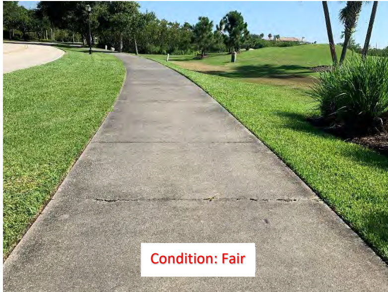
(231) Center Crack and Chipped Concrete
