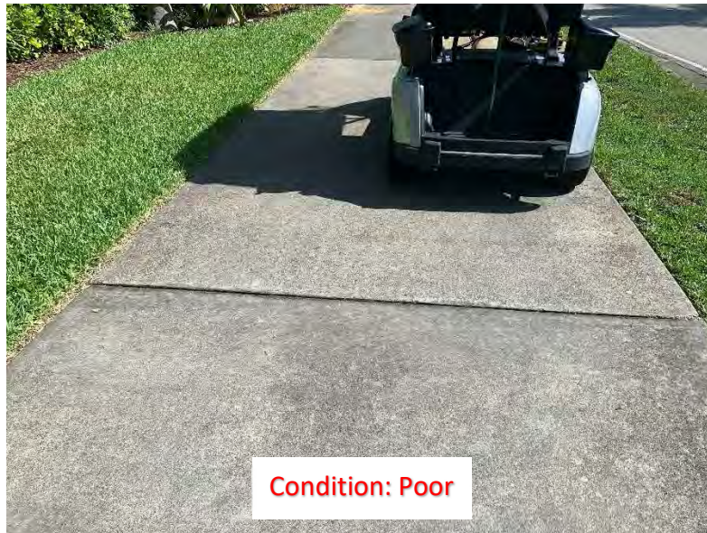
(242) Elevated Corners and Corner Crack (1)
