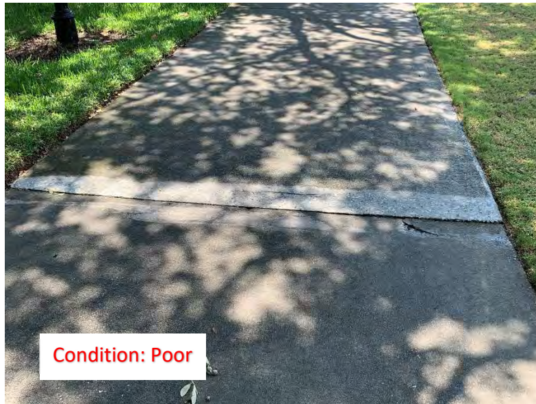
(127) Elevated Corners and Corner Cracks
