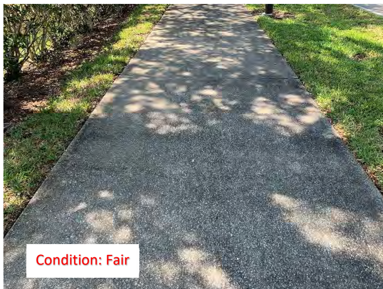
(105) Elevated Corner and Center Crack
