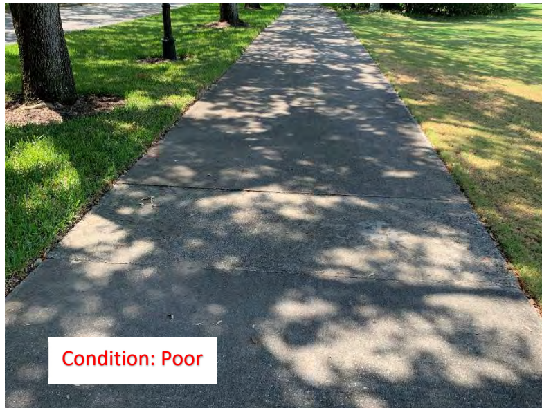
(140) Elevated Corners, Corner and Center Cracks (3)
