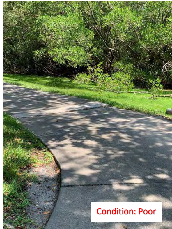
(143) Elevated Corners, Corner and Center Cracks (7)
