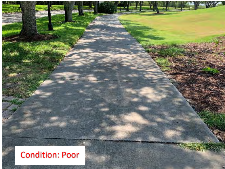
(123) Elevated Corner and Center Cracks
