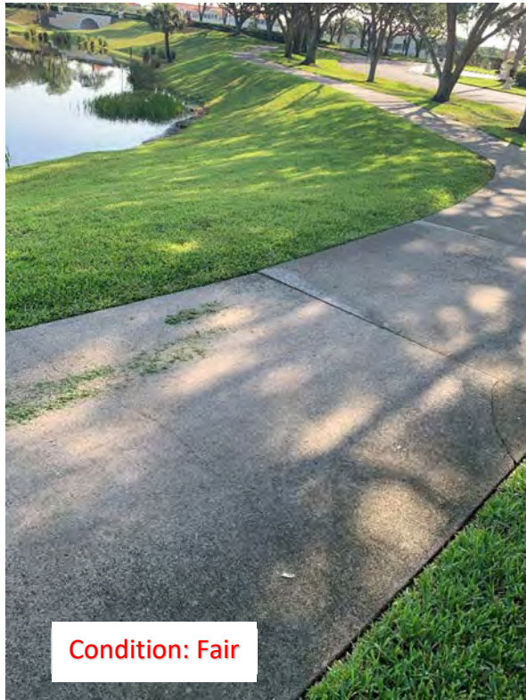
(20) Elevated Corner, Corner and Center Cracks
