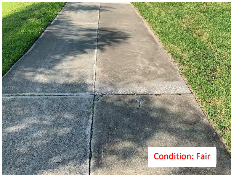
(80) Corner and Center Cracks
