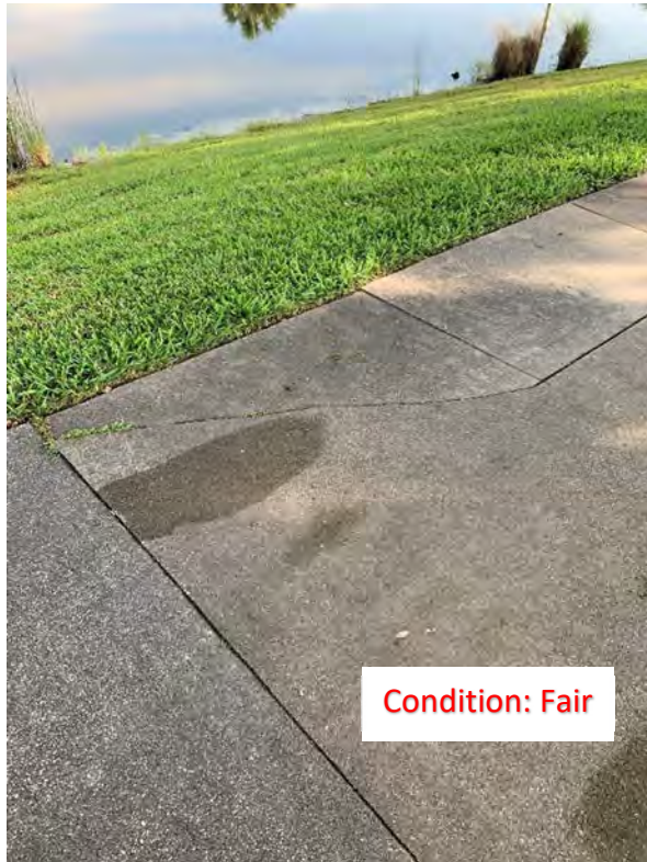
(26) Elevated Corner, Corner and Center Cracks (2)
