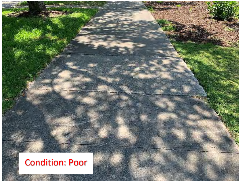
(122) Elevated Corners, Corner and Center Cracks (1)
