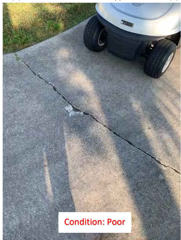
(5) Center Cracks and Chipped Concrete (3)
