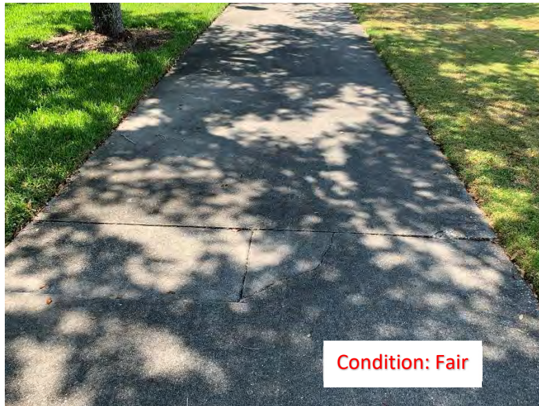
(138) Elevated Corners, Corner and Center Cracks
