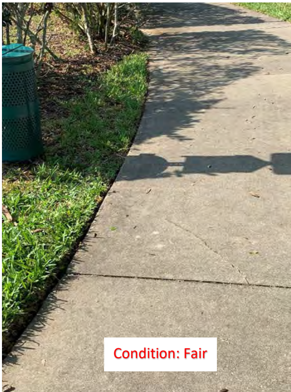
(88) Center and Corner Cracks
