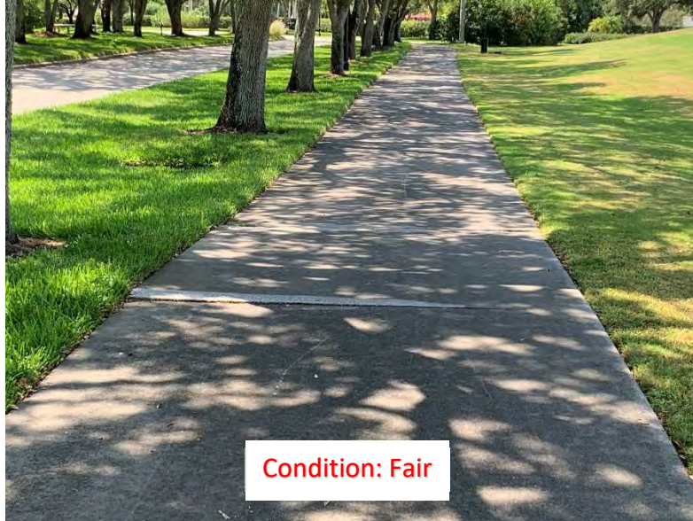
(137) Elevated Corners and Corner Cracks (1)
