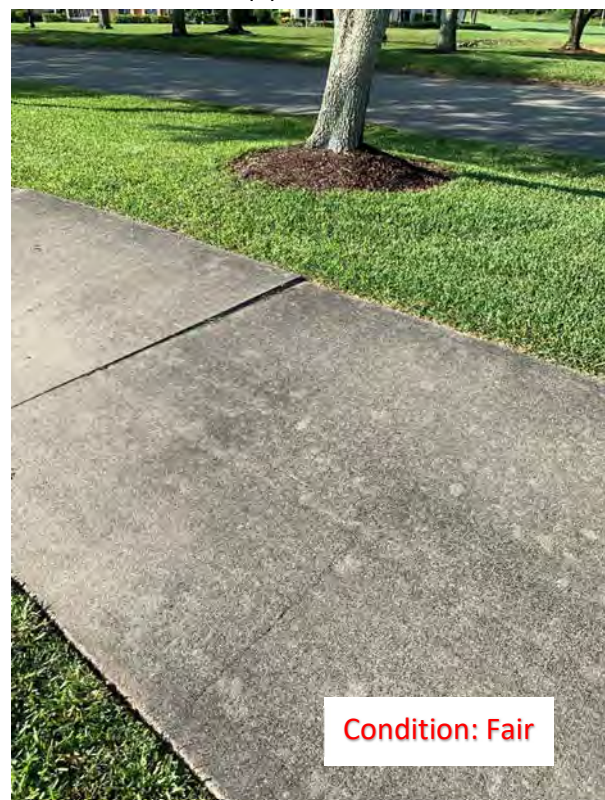
(11) Elevated Corner and Center Crack
