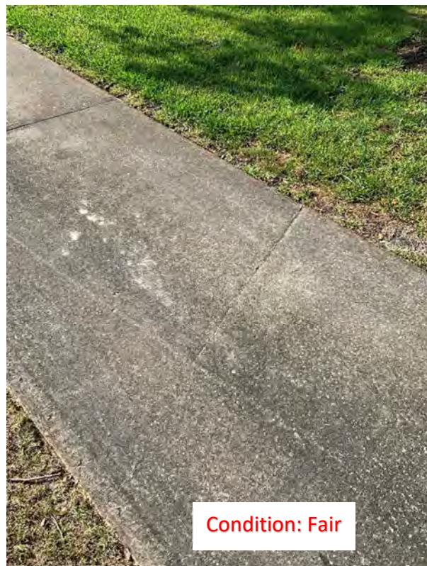
(53) Elevated Corner and Center Crack (2)
