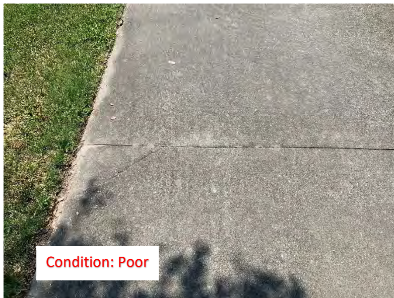
(143) Elevated Corners, Corner and Center Cracks (6)
