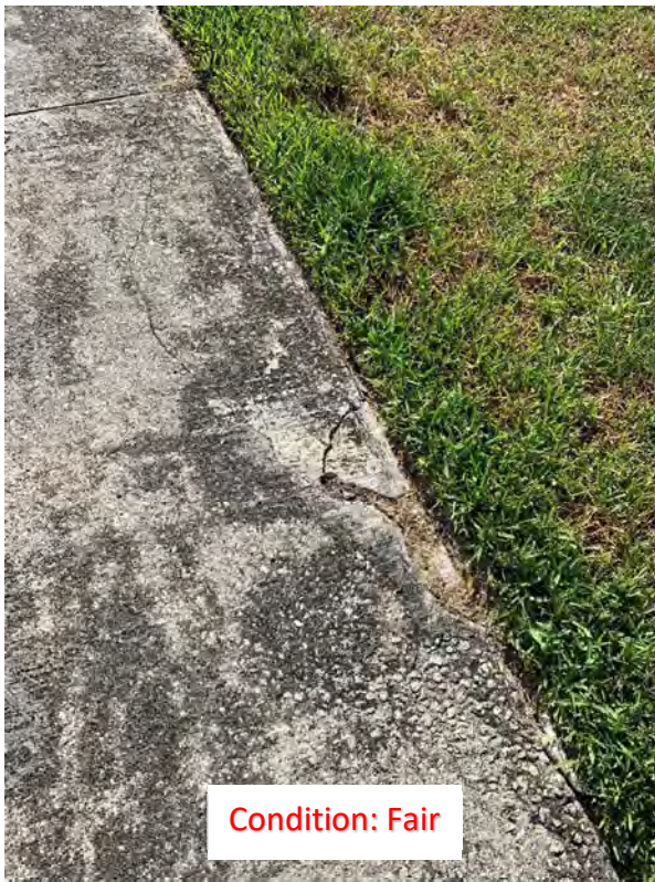
(50) Corner Cracks and Chipped Concrete (2)
