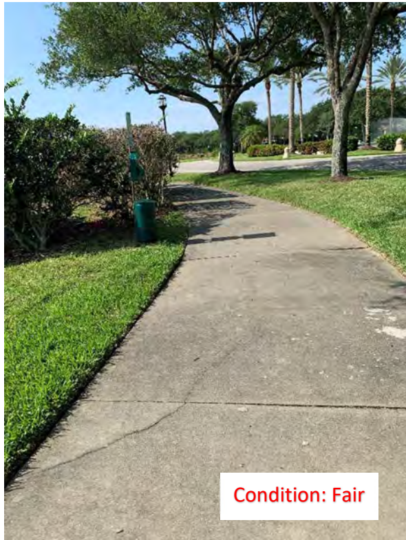
(88) Center and Corner Cracks
