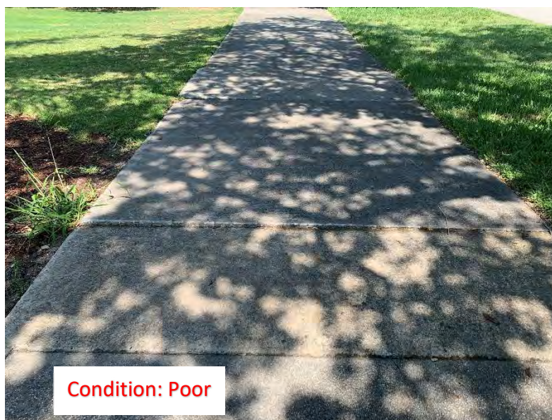
(122) Elevated Corners, Corner and Center Cracks (2)
