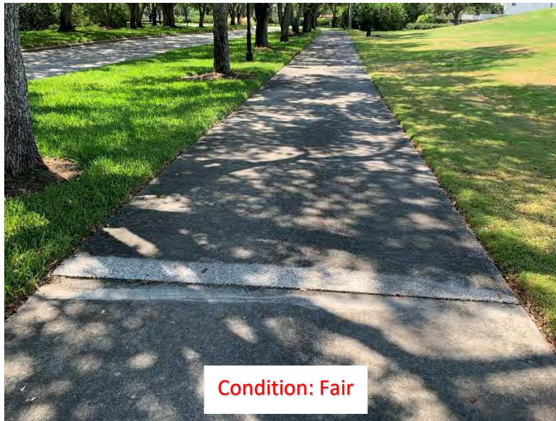
(137) Elevated Corners and Corner Cracks (1)
