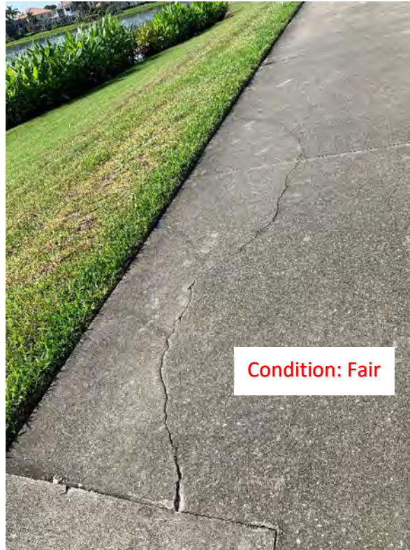
(86) Center and Corner Cracks
