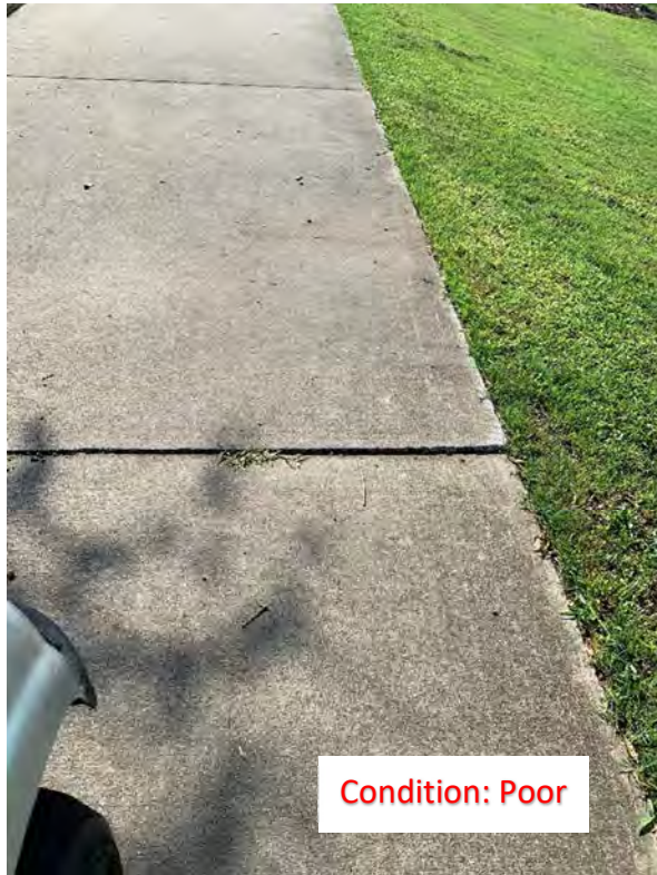
(64) Elevated Corner and Corner Crack (1)
