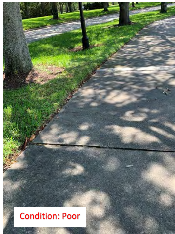
(127) Elevated Corners and Corner Cracks
