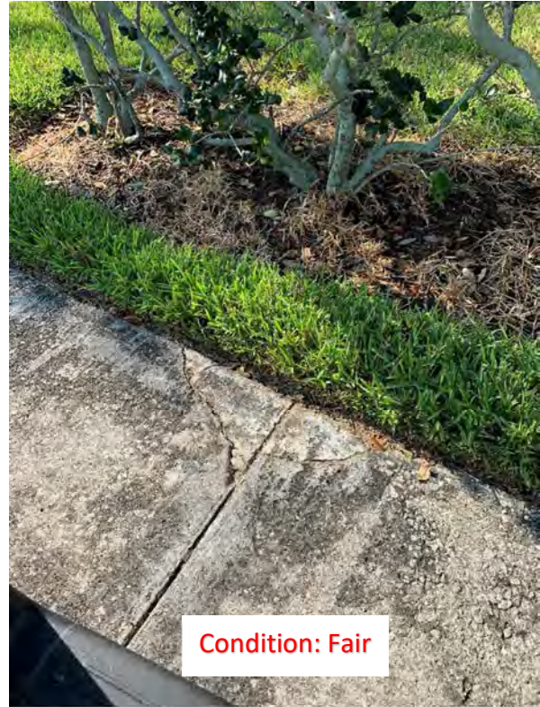
(50) Corner Cracks and Chipped Concrete (1)
