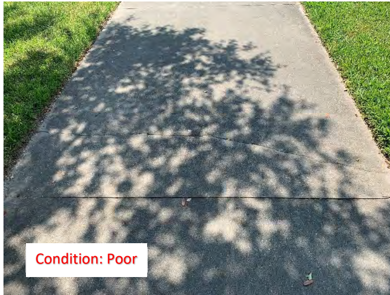
(143) Elevated Corners, Corner and Center Cracks (5)
