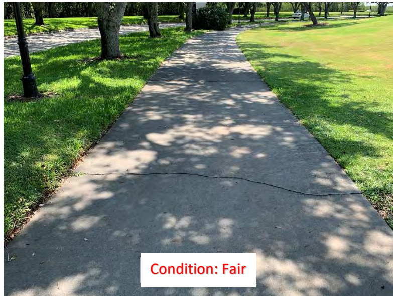
(125) Elevated Corner and Center Cracks
