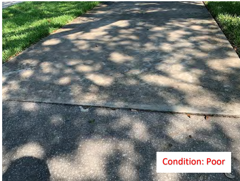
(99) Elevated Corners and Center Crack
