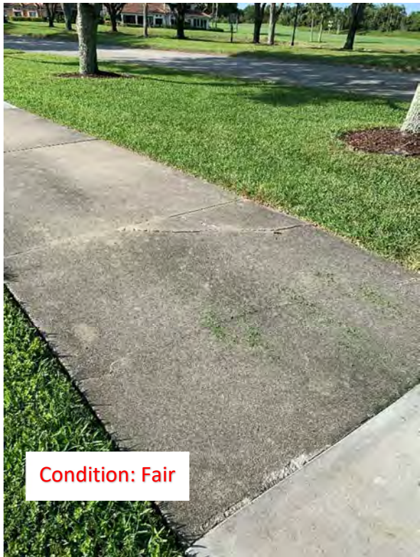
(7) Corner and Center Cracks
