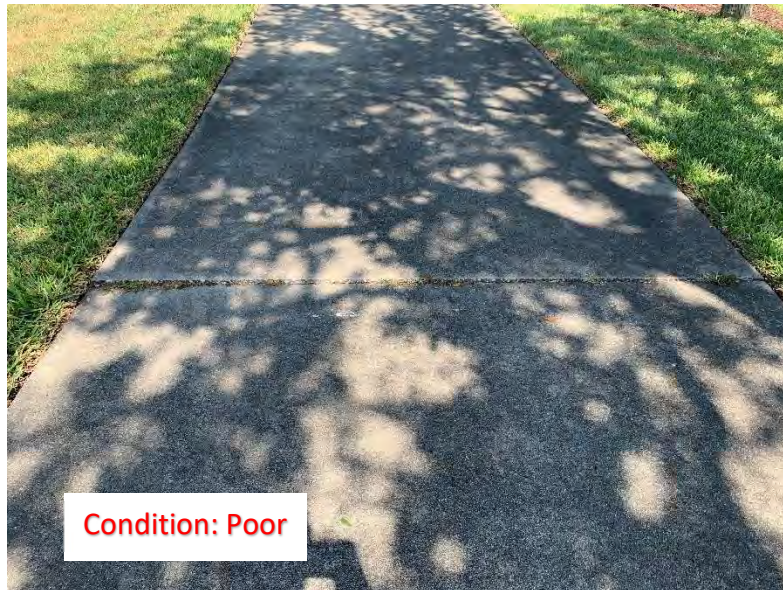
(115) Elevated Corner and Center Crack (1)
