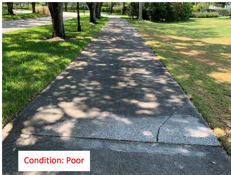
(140) Elevated Corners, Corner and Center Cracks (2)
