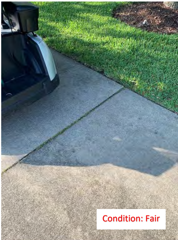
(14) Elevated Corner and Corner Crack
