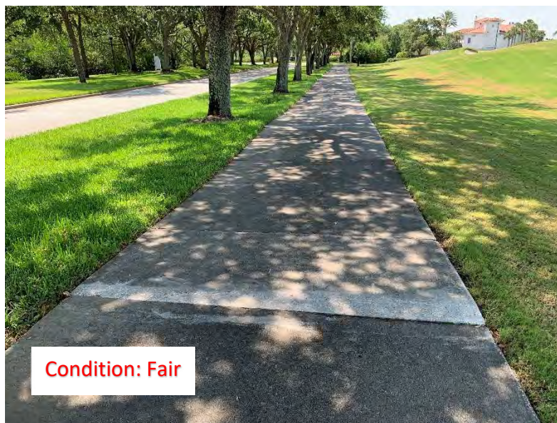
(136) Elevated Corners and Corner Cracks
