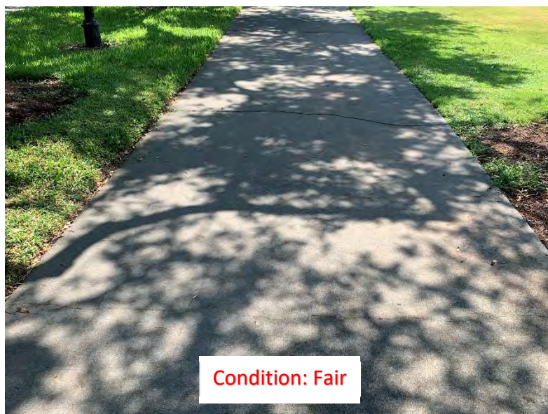
(124) Elevated Corner and Center Cracks
