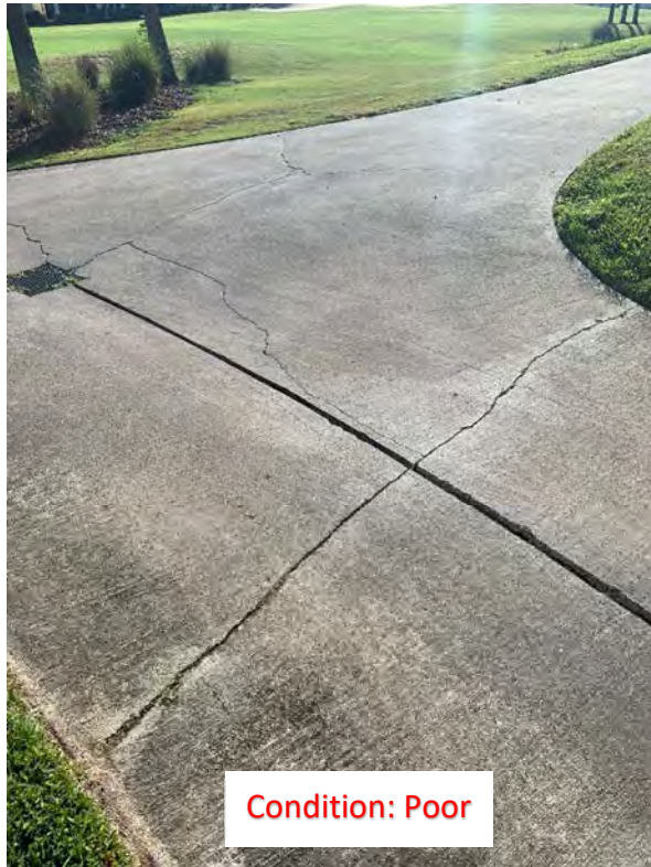
(5) Center Cracks and Chipped Concrete (4)
