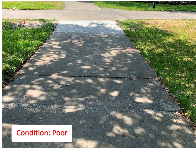
(140) Elevated Corners, Corner and Center Cracks (5)
