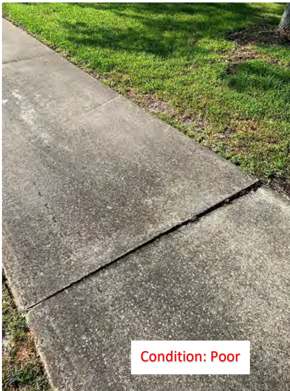
(53) Elevated Corner and Center Crack (1)
