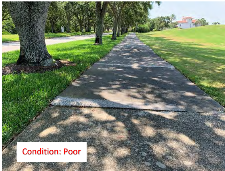
(135) Elevated Corners and Center Cracks
