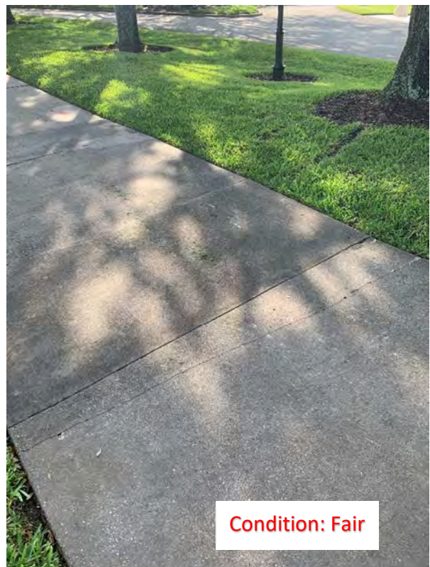
(29) Elevated Corner, Corner and Center Cracks
