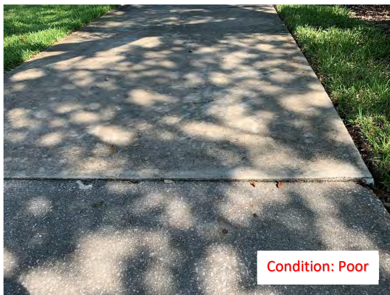
(100) Elevated Corner and Center Crack
