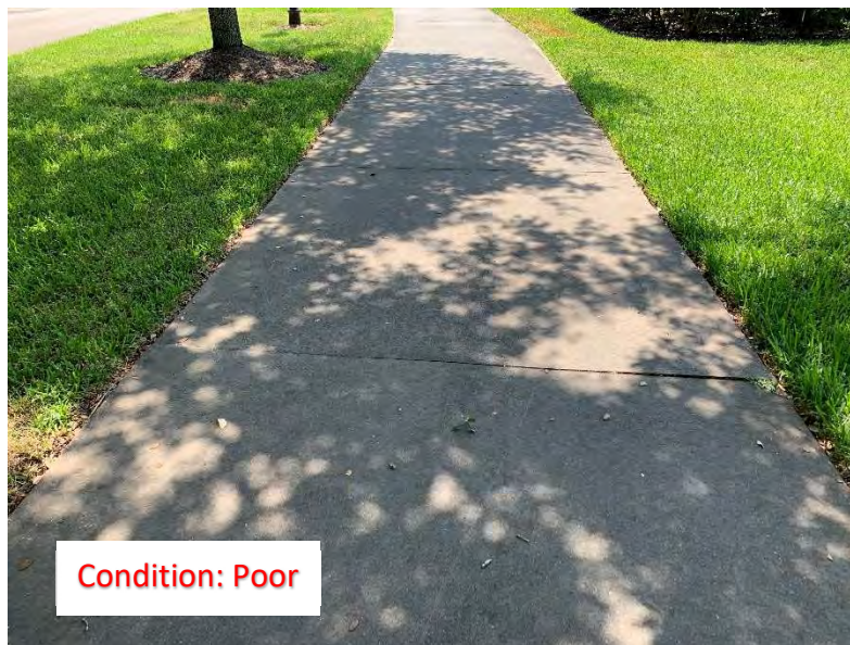
(143) Elevated Corners, Corner and Center Cracks (4)
