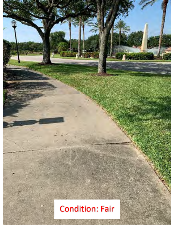
(88) Center and Corner Cracks
