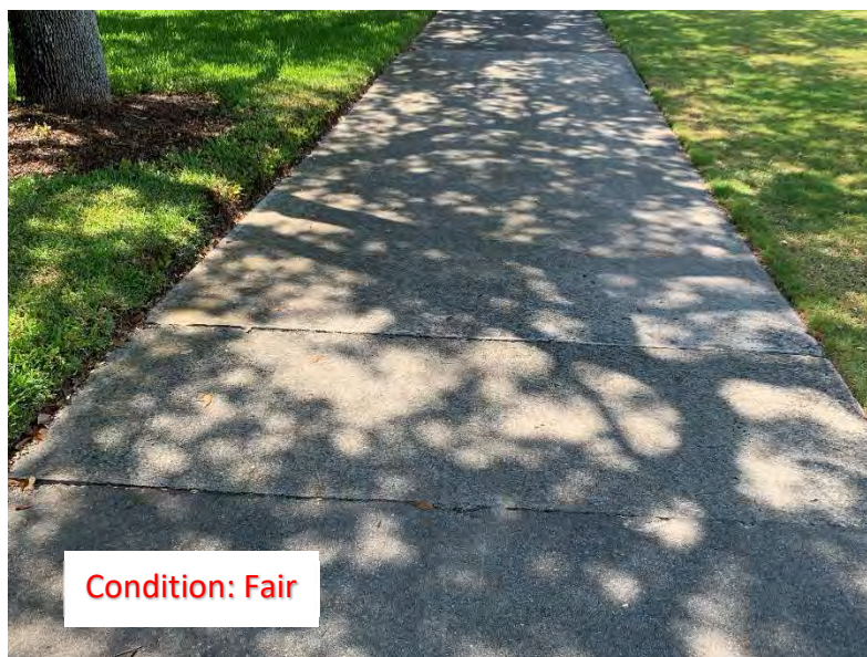
(139) Elevated Corners and Corner Cracks
