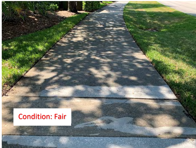
(117) Center Cracks and Corner Crack
