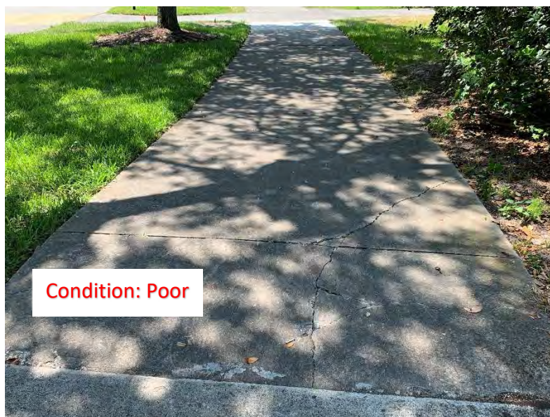
(140) Elevated Corners, Corner and Center Cracks (4)
