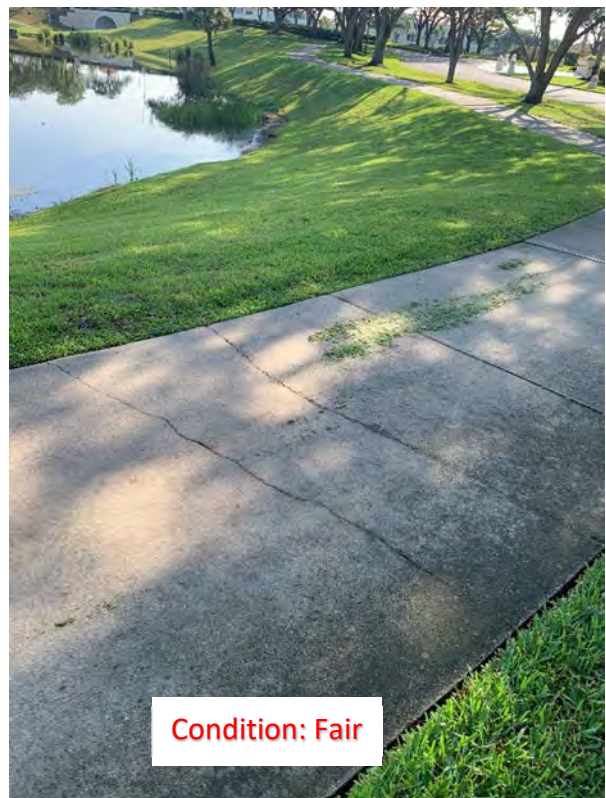
(19) Two Center Cracks
