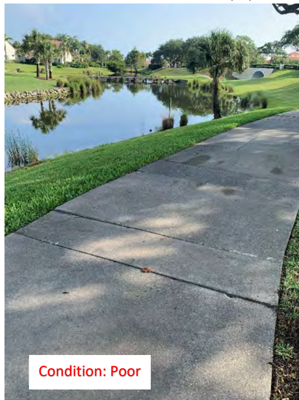
(26) Elevated Corner, Corner and Center Cracks (1)
