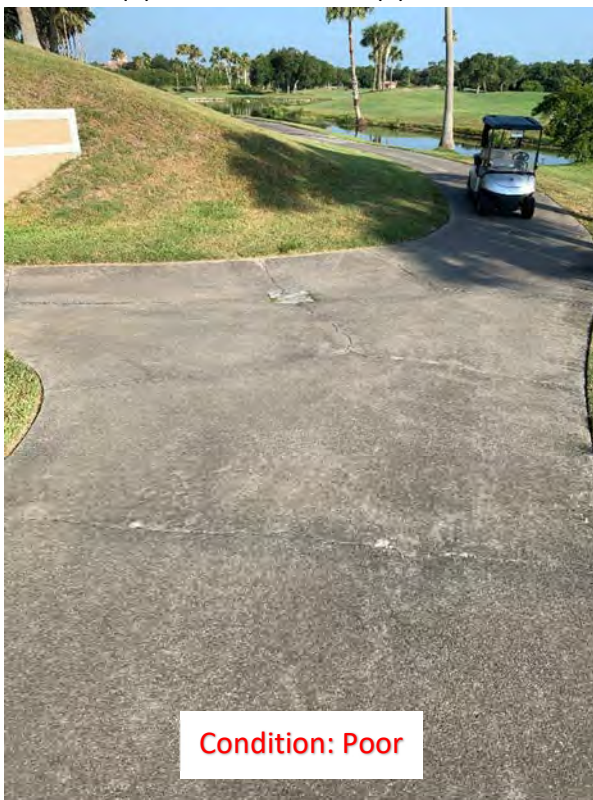
(5) Center Cracks and Chipped Concrete (2)
