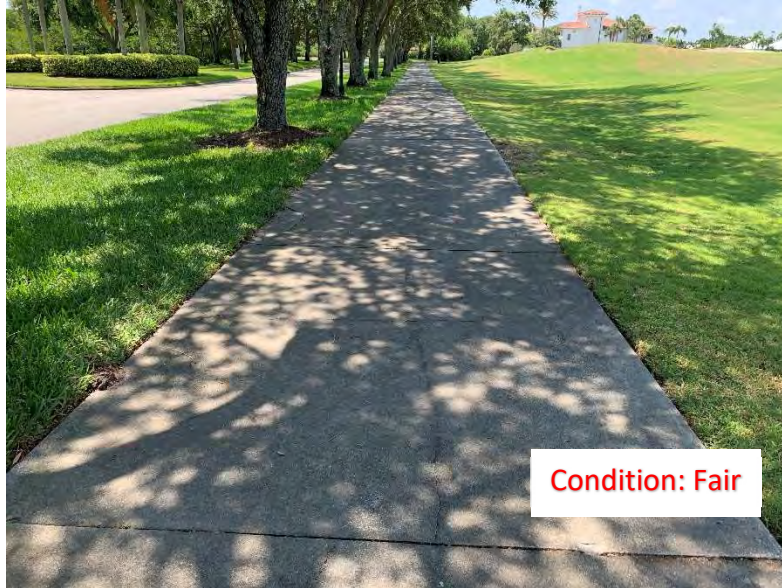
(132) Center and Side Cracks (1)
