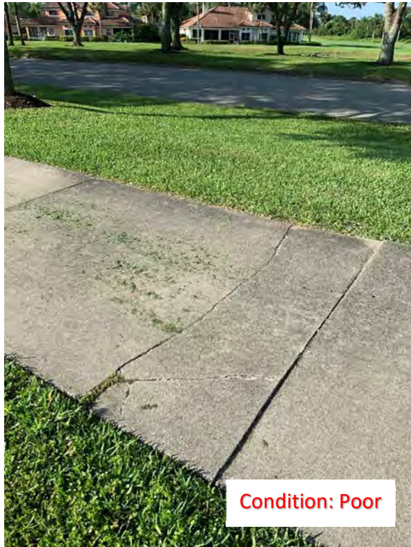
(12) Corner and Side Crack
