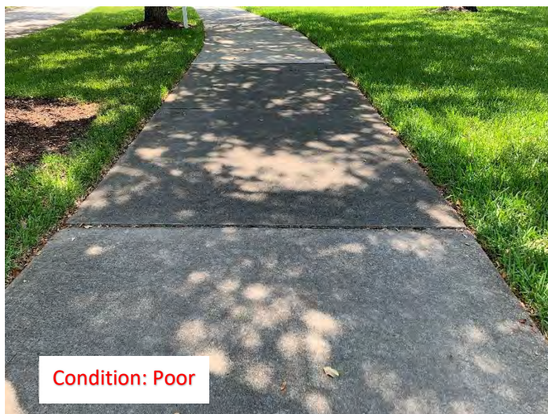
(143) Elevated Corners, Corner and Center Cracks (2)
