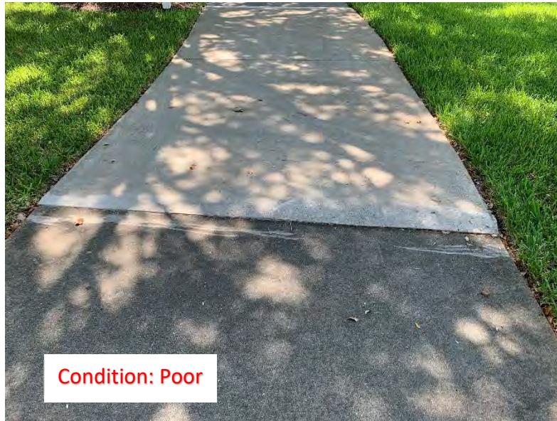
(143) Elevated Corners, Corner and Center Cracks (3)
