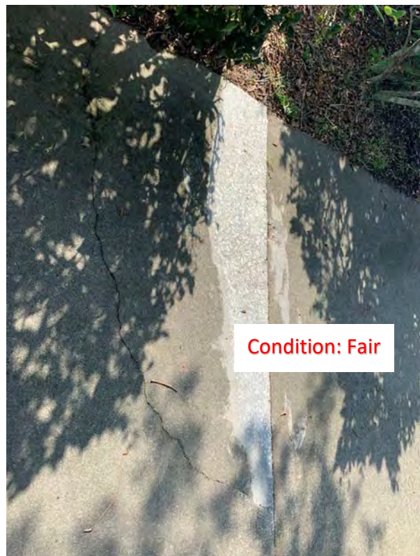
(88) Center and Corner Cracks
