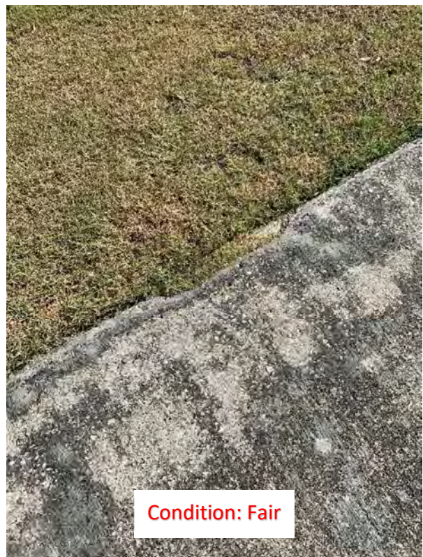
(50) Corner Cracks and Chipped Concrete (3)
