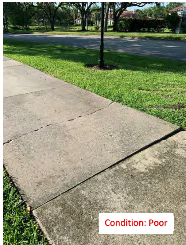
(15) Elevated Corner, Corner and Center Cracks
