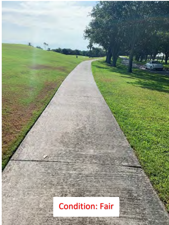
(51) Elevated Corner and Corner Crack
