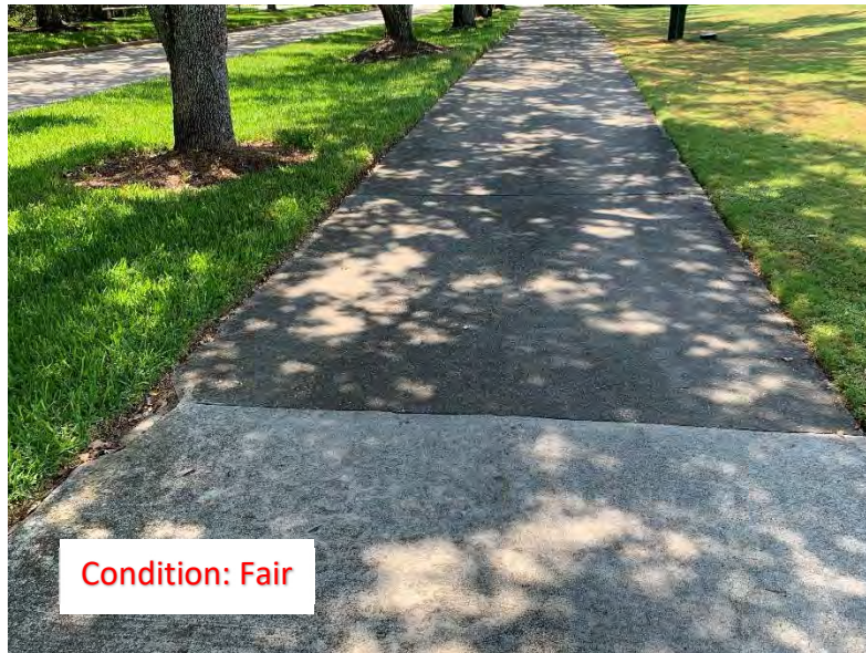
(140) Elevated Corners, Corner and Center Cracks (1)
