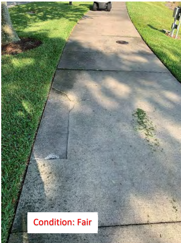
(18) Corner and Side Cracks
