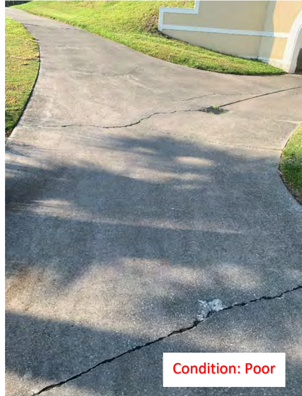
(5) Center Cracks and Chipped Concrete (1)
