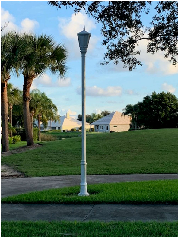
(1) Light Pole Off/Not Working
