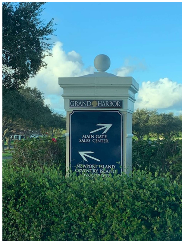
(8) Pillar Sign Light Off/Not Working
