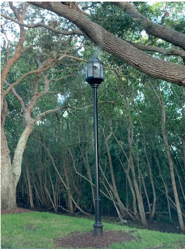
(7) Dim Light Pole
