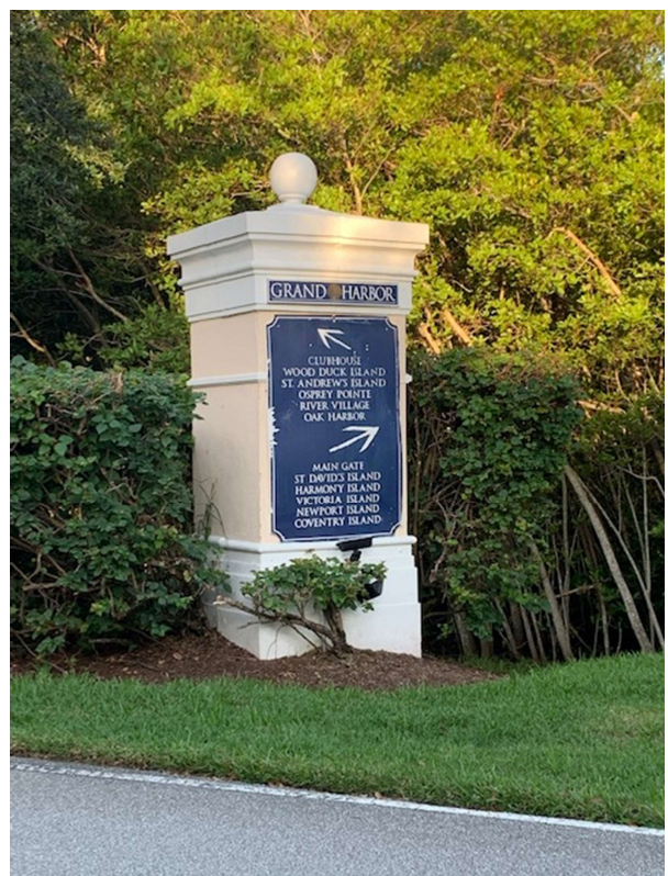
(4) Pillar Sign Light Off/Not Working
