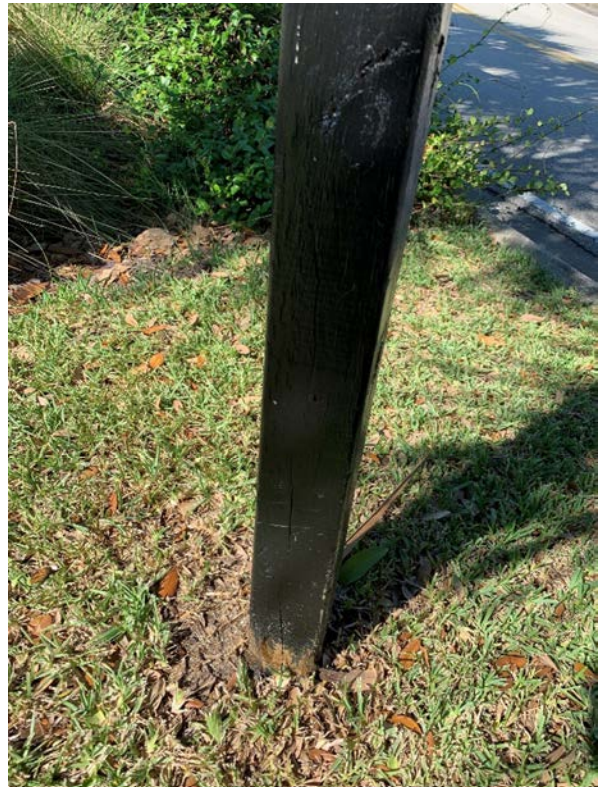
(27) Sign and Post Decay (2)
