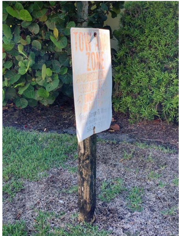
(29) Sign and Post Decay
