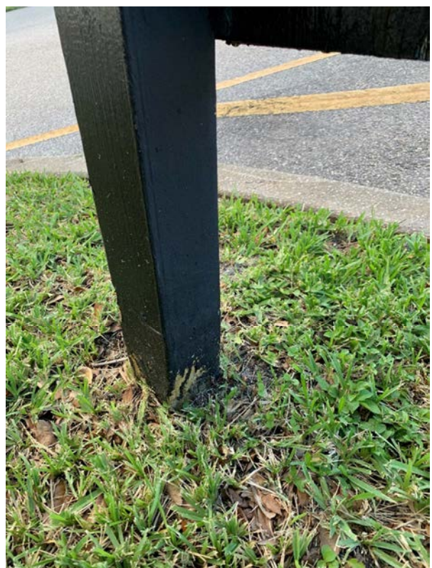
(2) Post Decay/Cracked Sign (2)
