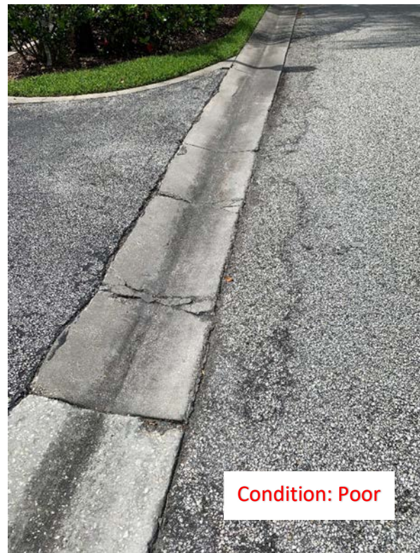
(8) Uneven Gutter/Gutter Crack
