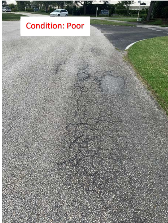
(46) Large Asphalt Cracks
