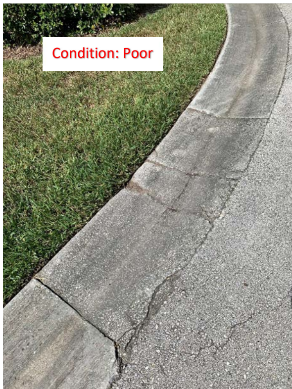
(1) Curb and Gutter Cracking (3)
