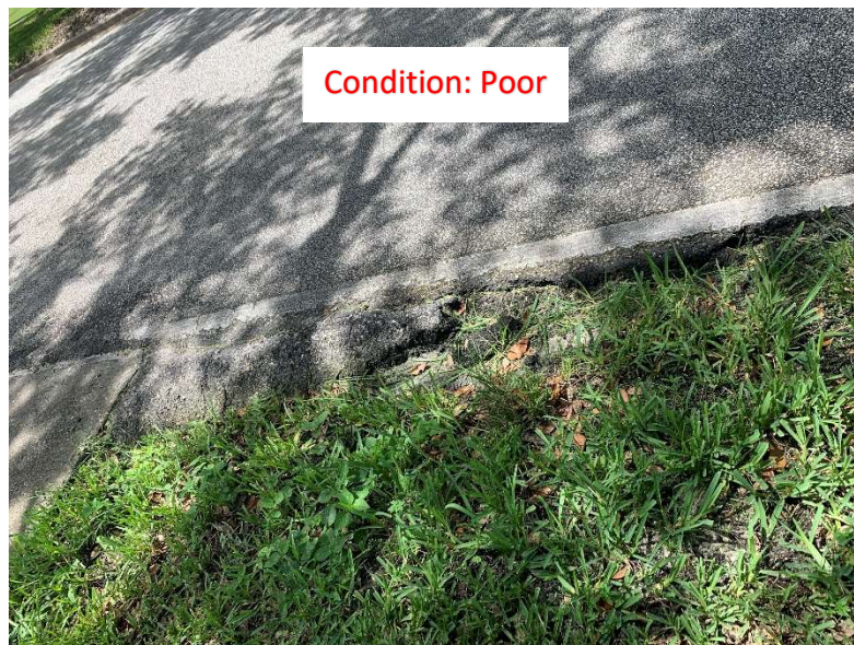
(50) Collapsed Asphalt Areas
