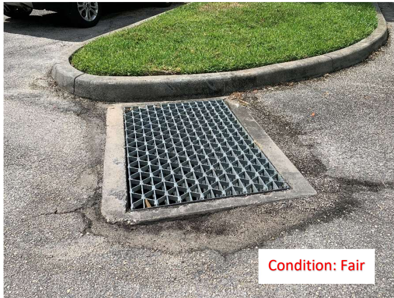
(16) Dip Around Grate Inlet
