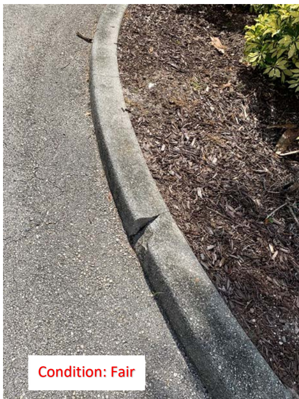
(3) Curb Cracking and Chipping (3)
