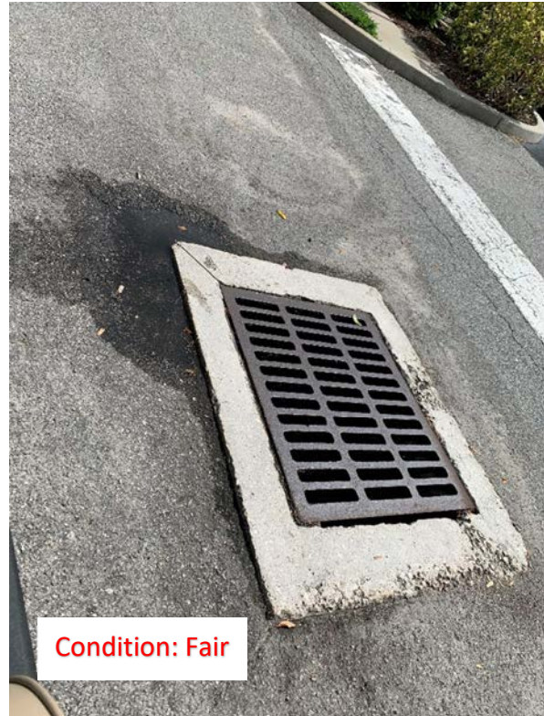
(20) Dip Around Grate Inlet
