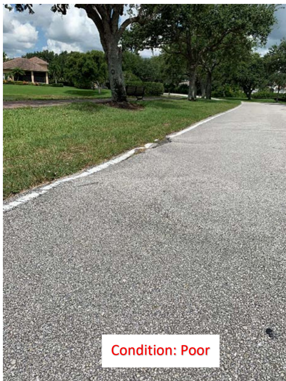
(24) Large Significant Dips/Cracking
