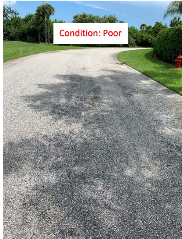
(23) Large Area Significant Cracking
