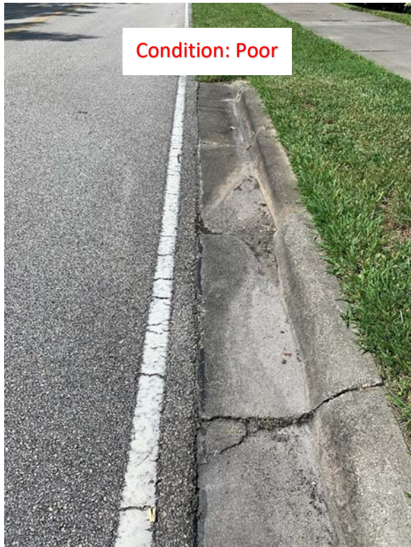
(1) Curb and Gutter Cracking (1)
