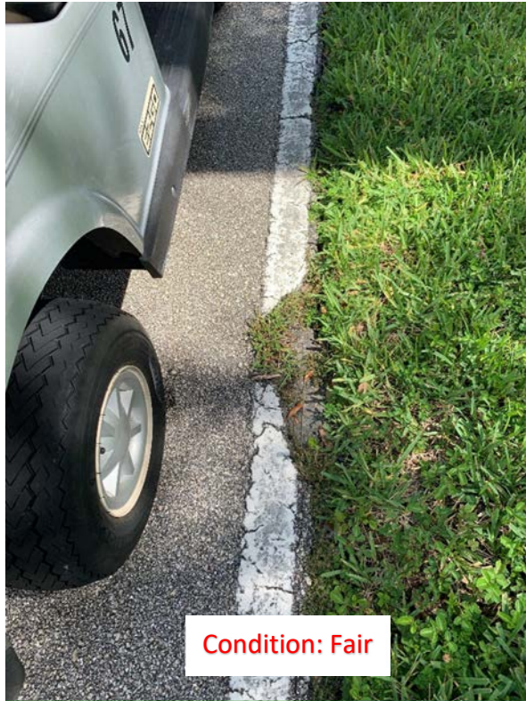
(5) Small Asphalt Collapse
