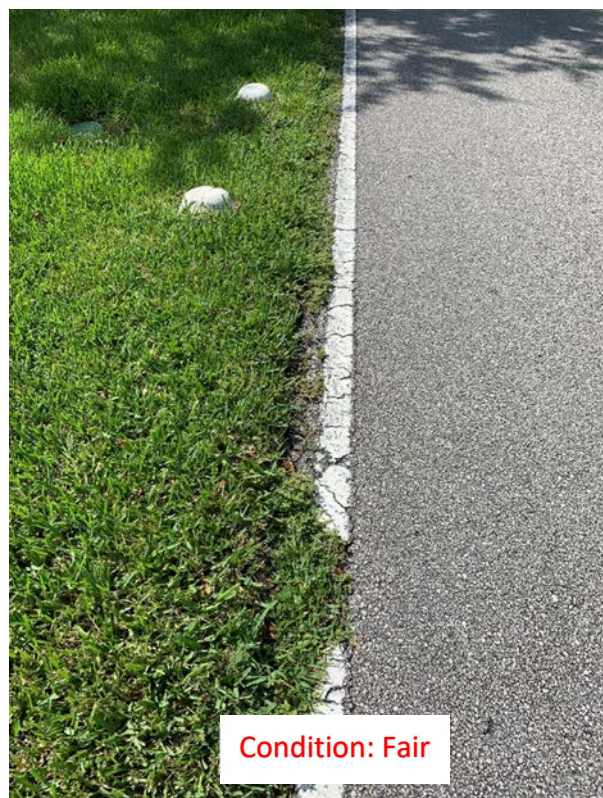
(4) Small Side Collapse
