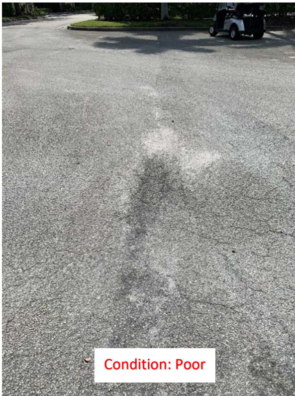
(7) Large Dip and Significant Cracking
