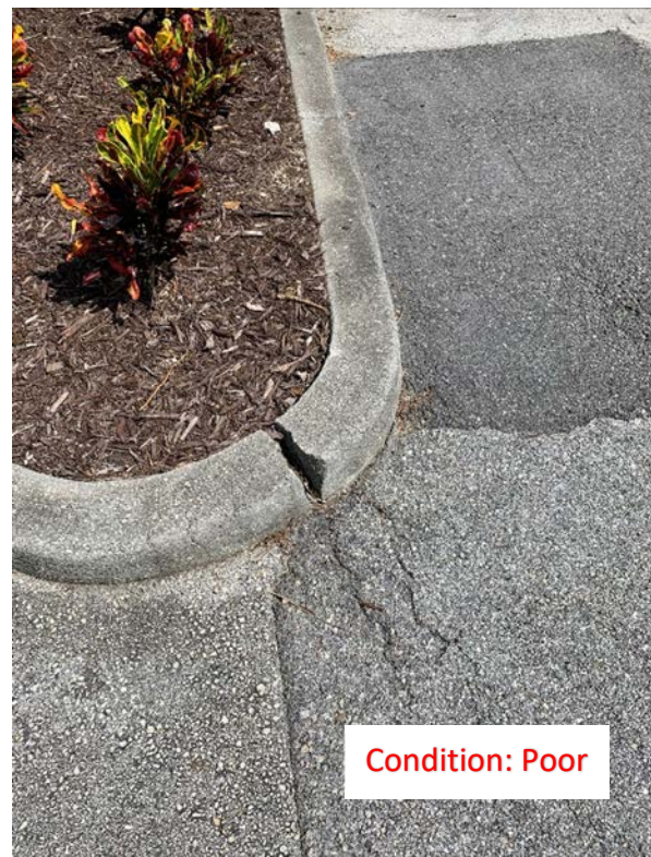
(2) Large Curb Crack
